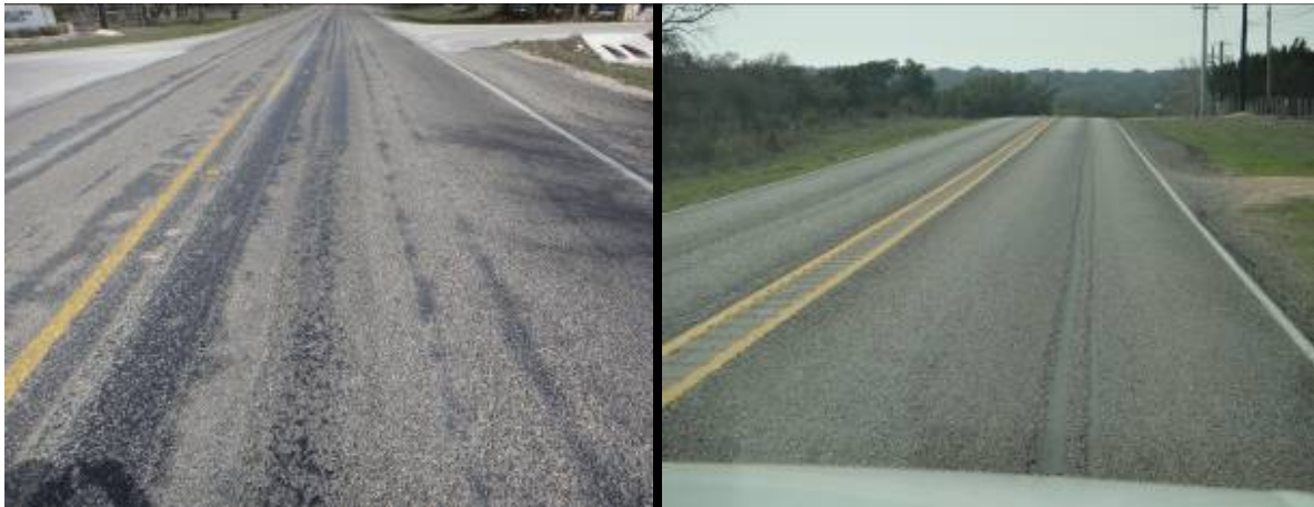
Figure 1. Poorly Performing Seal Coat on RM 12.
