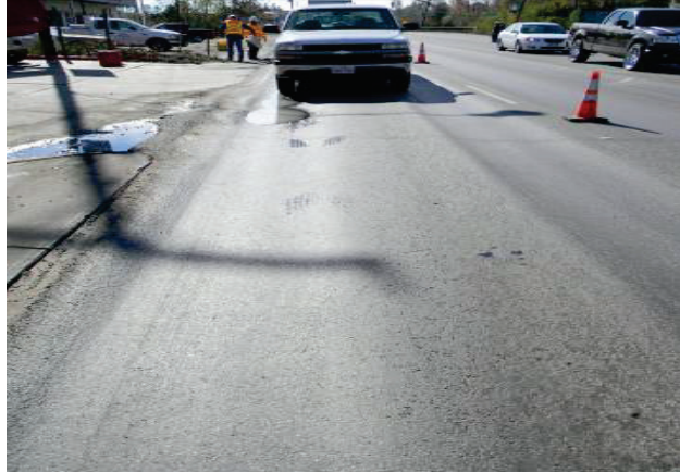
Figure 1-2. Severe Surface Rutting on US 96 in Beaumont District (over 1.5 inch Rut Depth).
