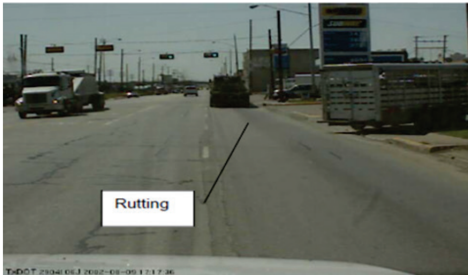
Figure 1-3. Surface Rutting on Anderson Street in Bryan District (over 0.5 inch Surface Rutting).
