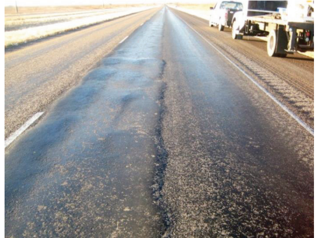
FIGURE 4 – Surface Stability Problems due to Multiple Chip Seals (Must Be Milled Prior to Placement of Thin Overlay).
