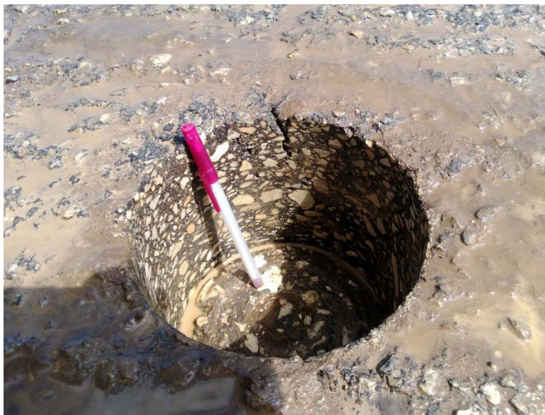
Figure 6.13. Cracking Isolated in the Top HMA Layer.
