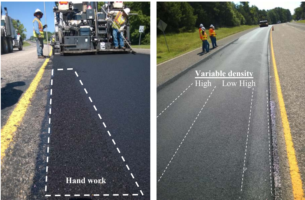
Figure G.11. Hand-Working Issue Causing Uneven Compaction.
