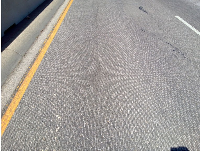
Figure 6.12. Low- to Moderate-Severity Block Cracking on Wurzbach Parkway.
