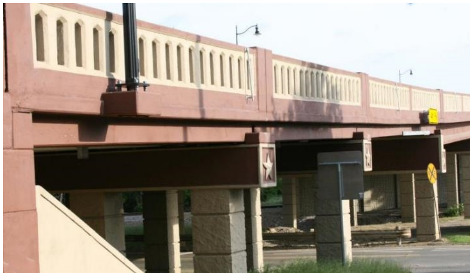
(b) Side View of Three Spread Slab Beam Spans (30 ft, 30 ft, and 50 ft Spans)
