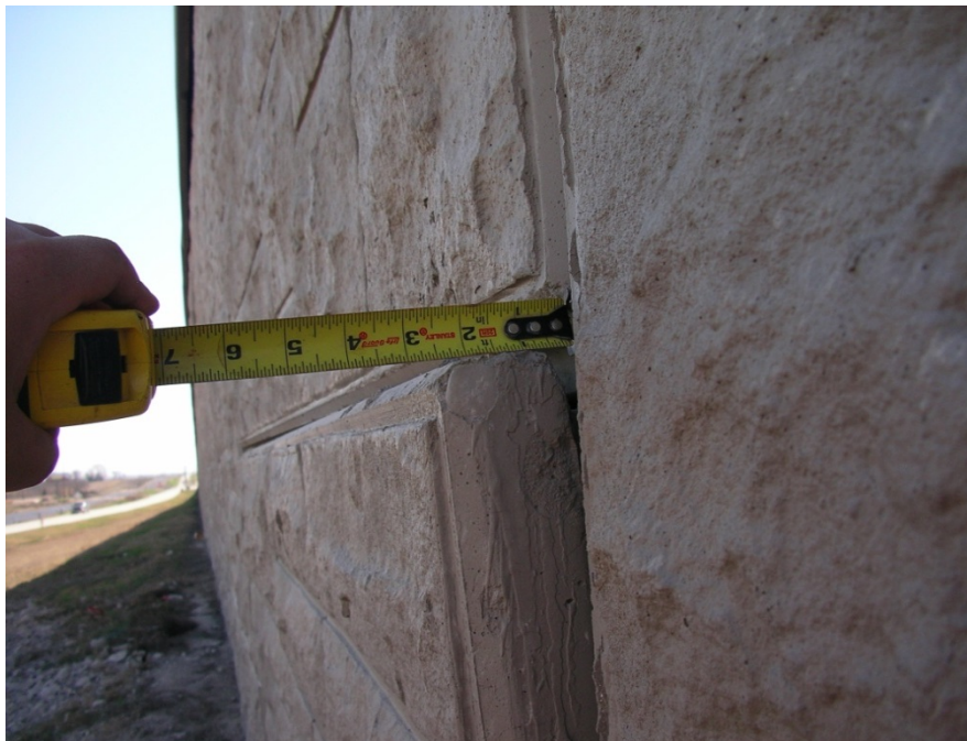
Figure 27. Dislocation of the MSE Wall Panels.
