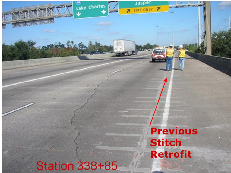
Figure 8. Recurring of Cracks on the Pavement.
