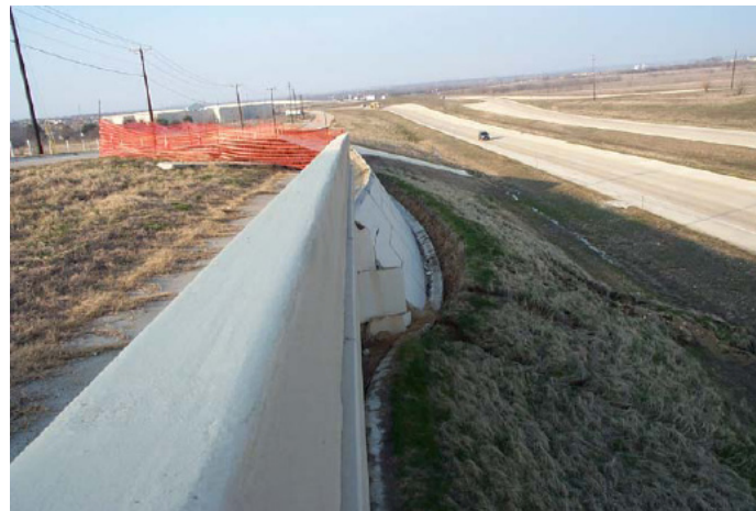
Figure 6. Example of MSE Wall Failure along the Slope.
