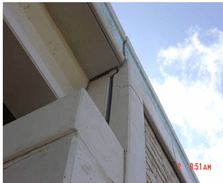
Figure 17. Outward Movement of Corner Panel at the Departure.
