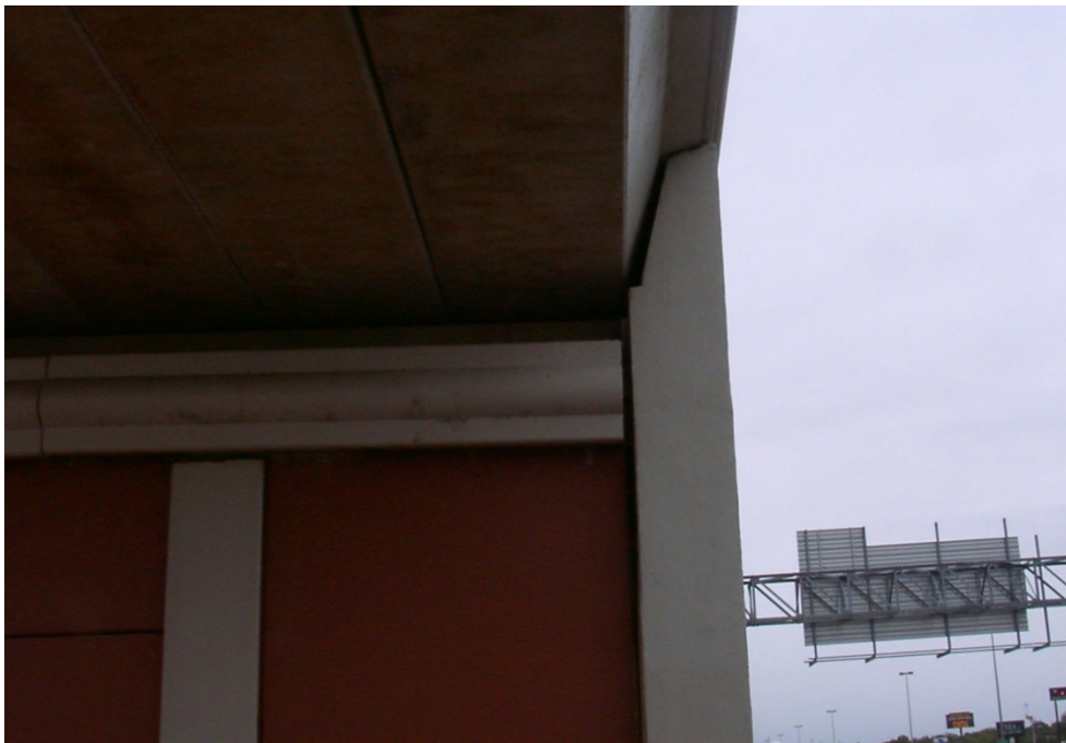
Figure 21. The Outward Movement of MSE Wall.
