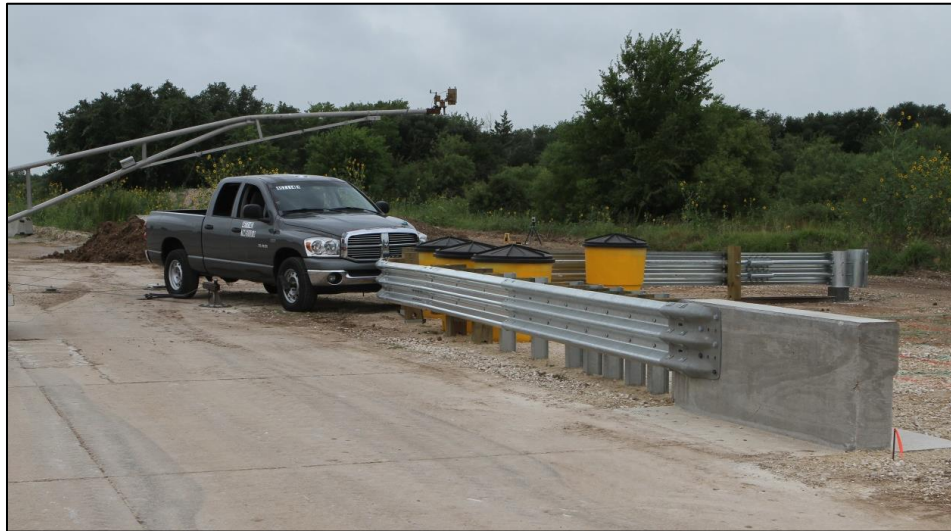
Figure 3. Short Radius Guardrail System.
