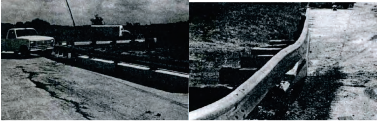
Figure 1.13. Impact Conditions and System Damage for YC-7 (3).
