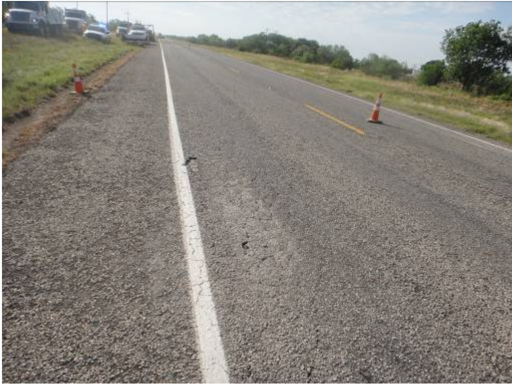
Figure 3.9 FM 55 Uvalde Isolated Location of Alligator Cracking in Surface Prior to LRA Application (of Martin Marietta Type D).
