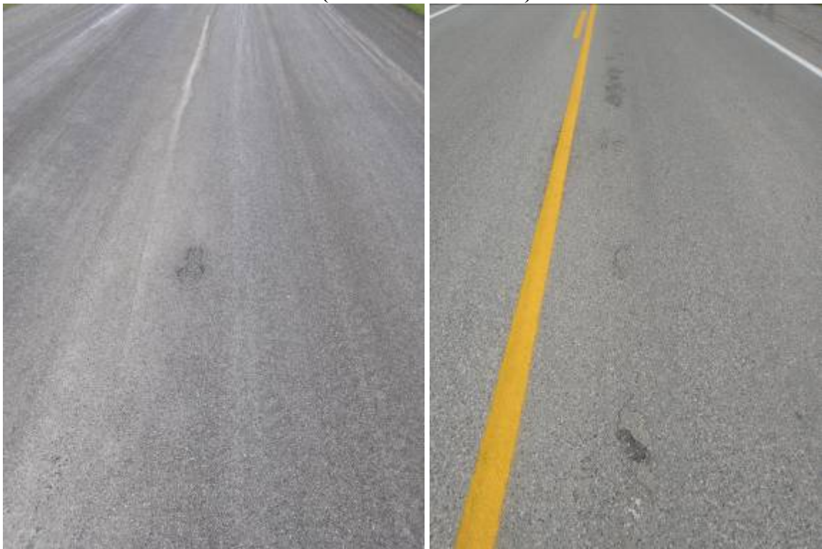
(b) Close up of Pothole (2 days After Rain) (c) Patched Potholes 3 months later. Figure 3.8. Jefferson Test Section Developed Pothole in Wheelpath in Area Holding Water (After a Rain in First Week).
