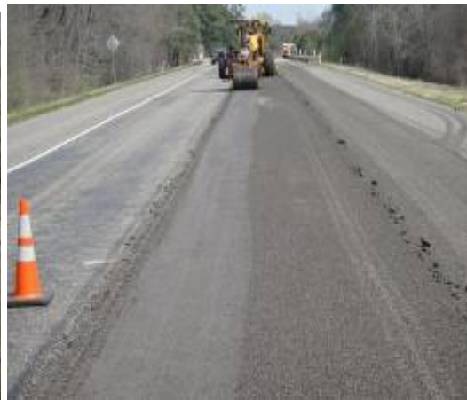
e) Steel Wheel Roller
