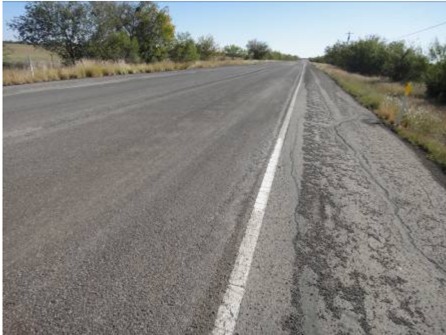
(a) Ravelling Observed 24 Hours After Construction.
