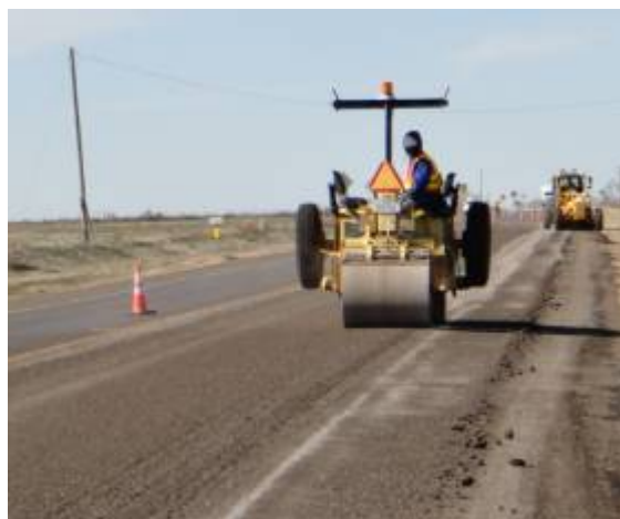
e) Steel Wheel Roller
