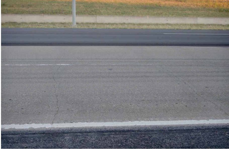
Figure 2-18. Existing Pavement Condition of Loop 820 Test Sections.
