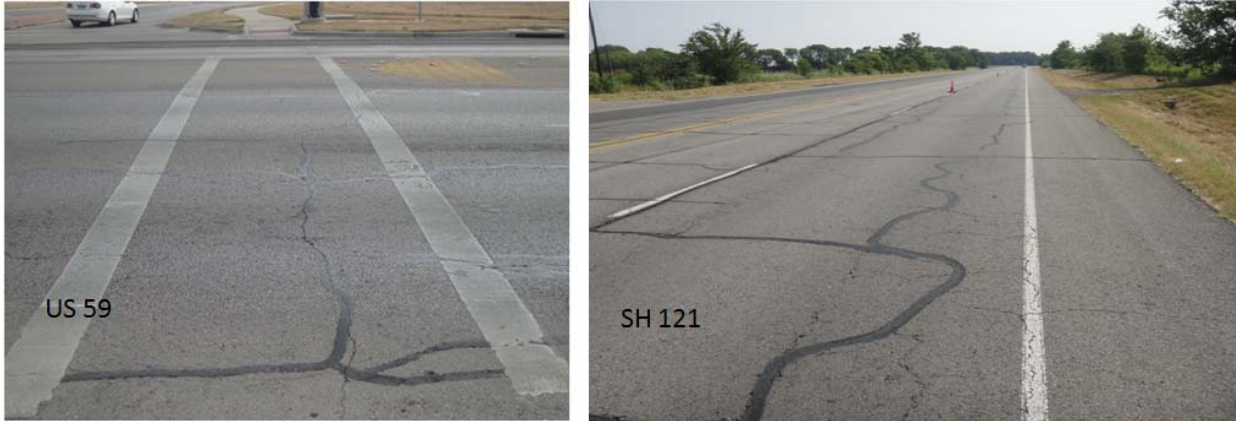
Figure 5-3. Cracking on US 59 (Atlanta District) and SH 121 (Paris District) Prior to Overlay Placement in Spring 2011.
