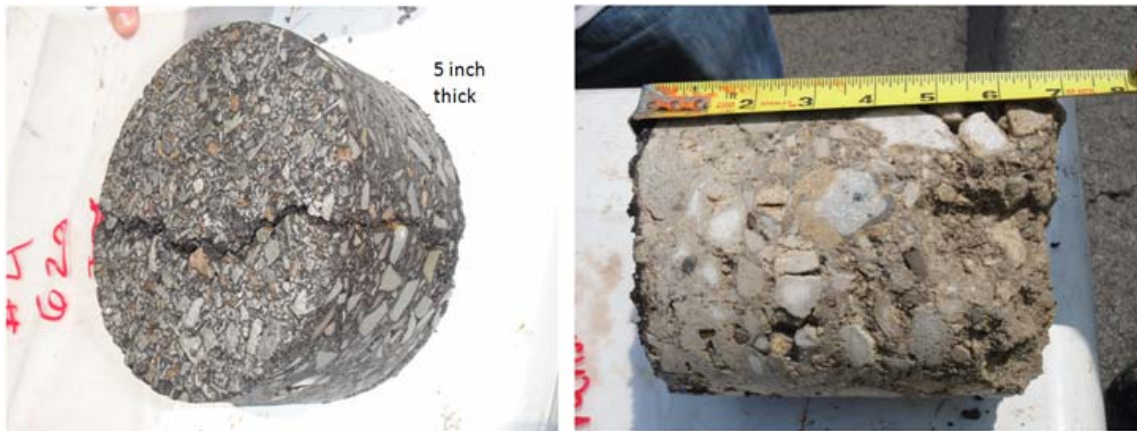
Figure 7-4. Cores from SH 121 (Paris District) Prior to Overlay.
