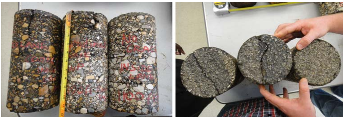
Figure 7-2. Defective Cores from US 59 (Atlanta District) Prior to Overlay.
