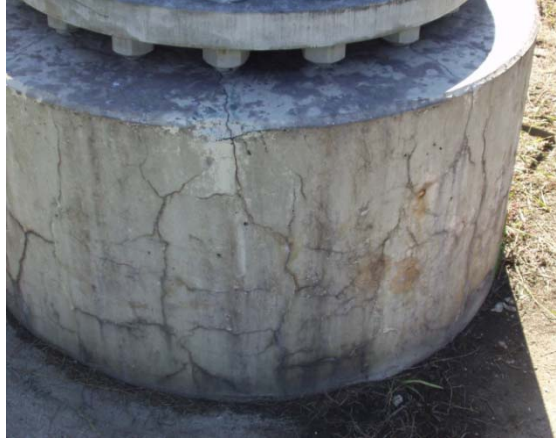
Figure 2.3. ASR Cracking in Cast-in-Place Elements.
