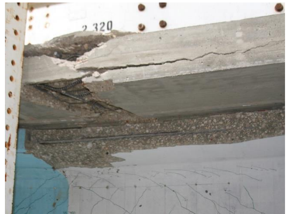
(e) Buckling of Longitudinal Bars in Deck
