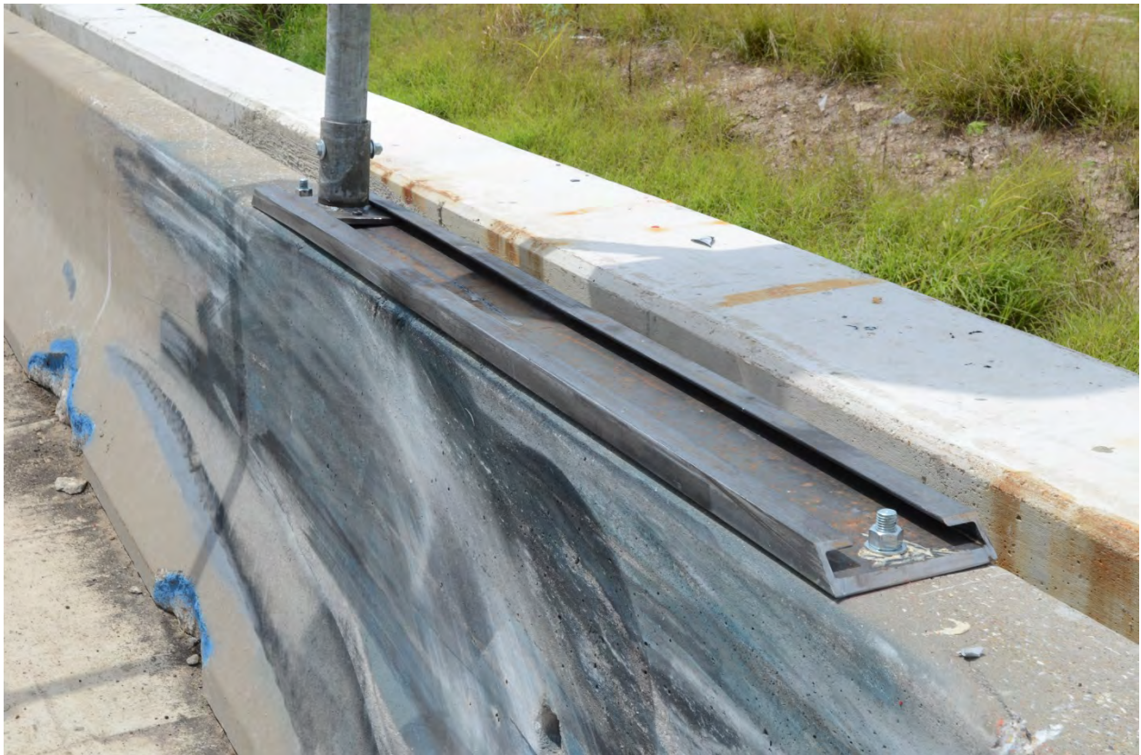
Figure 6.27. Chute Channel Sign Support on CMB after Test No. 466462-3.
