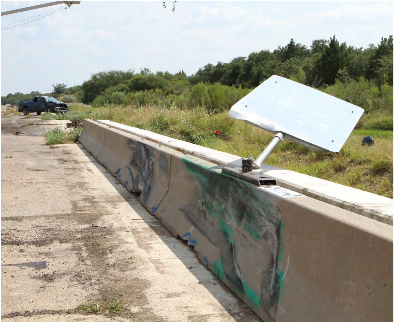
Figure 6.35. Vehicle/Slotted 10 BWG Sign Support on CMB after Test No. 466462-4.
