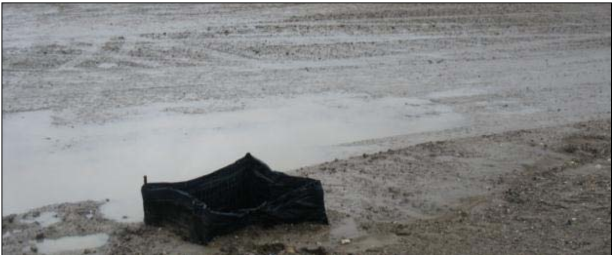
Figure 18. CS Project Watershed 3 Relatively Flat Drainage Area with Loose Bare Soil.
