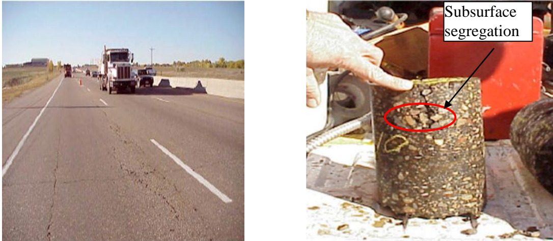
Figure 2-14. Top-Down Cracking on I-25, Colorado (after Harmelink et al. 2008).
