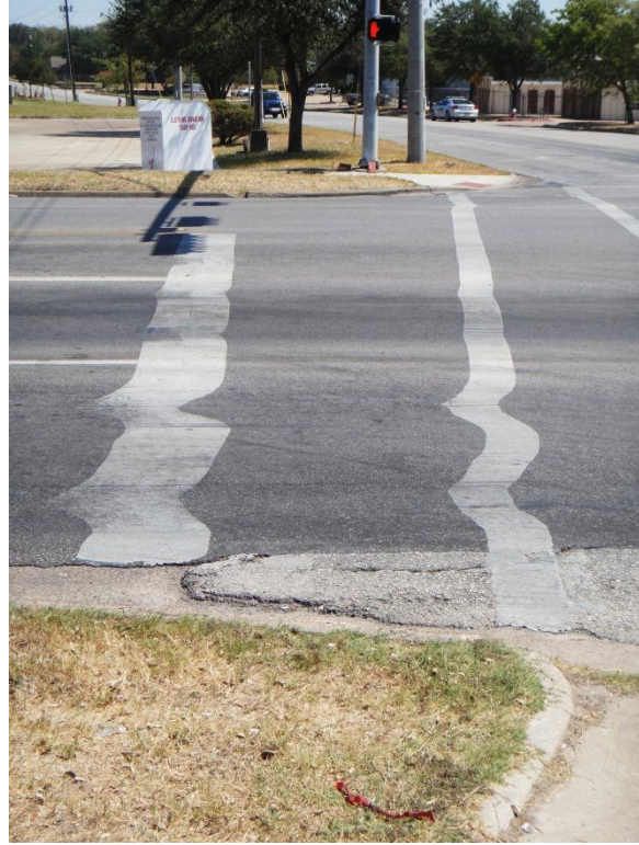
(b) Rutting and Shoving at the Stop Light
