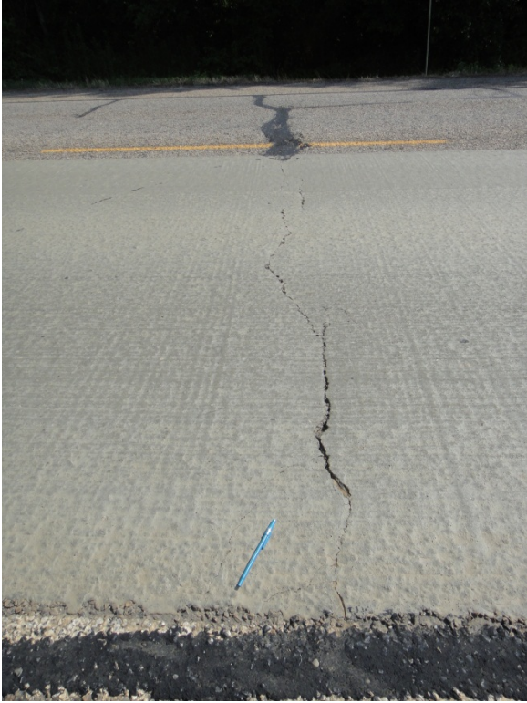
(a) Transverse Cracking
