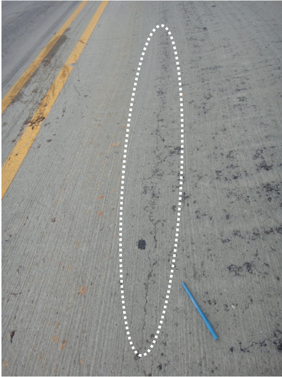
(a) Longitudinal Cracking
