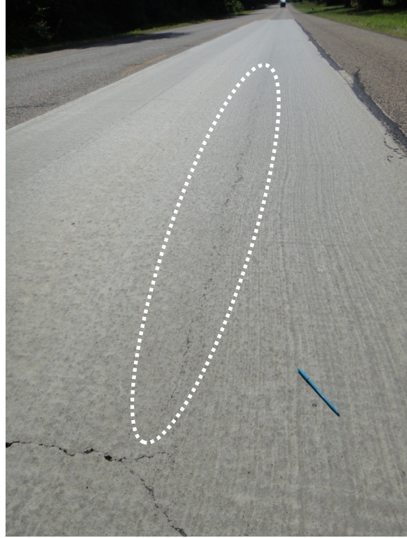
(b) Longitudinal Cracking
