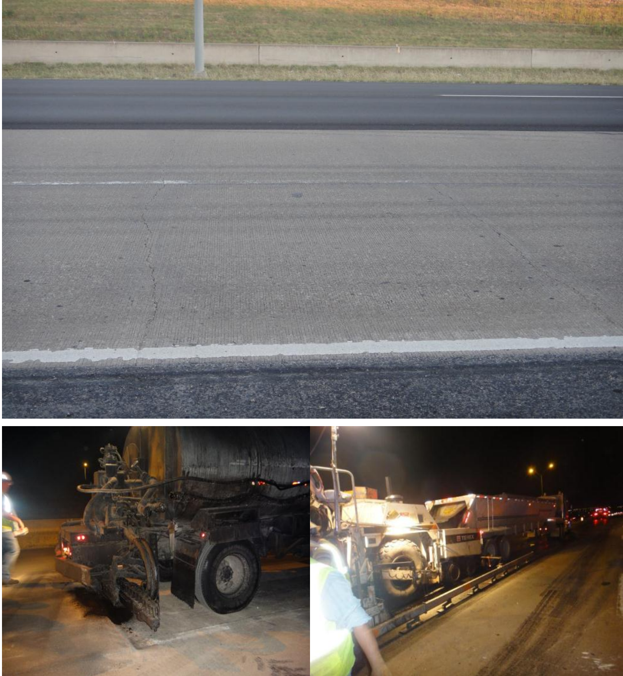
Figure 39. Existing CRCP Condition and Construction of RAP/RAS Test Sections on Loop 820, Fort Worth.
