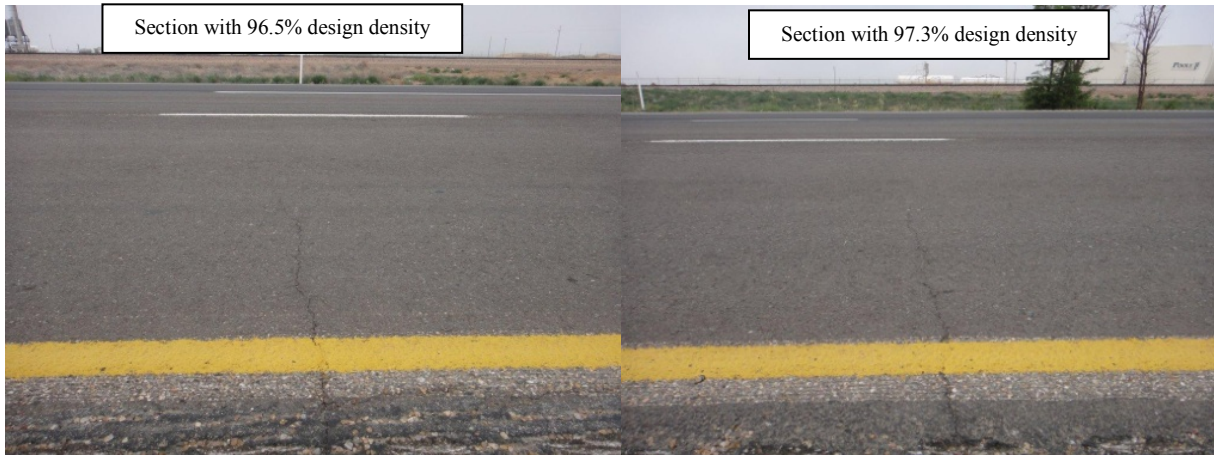
Figure 35. Observed Reflective Cracking of RAS Test Sections on US87, Amarillo, Texas.
