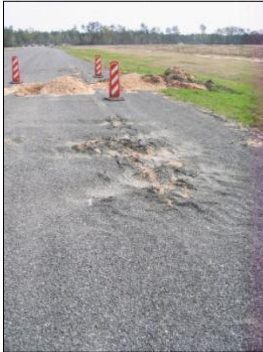
Figure 1.3. Base Failure during Construction where Base Accepted at 95 Percent Density.
