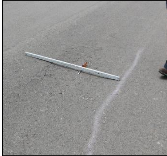
Figure 1.4. Premature Failure where 100 Percent Density Was Achieved.
