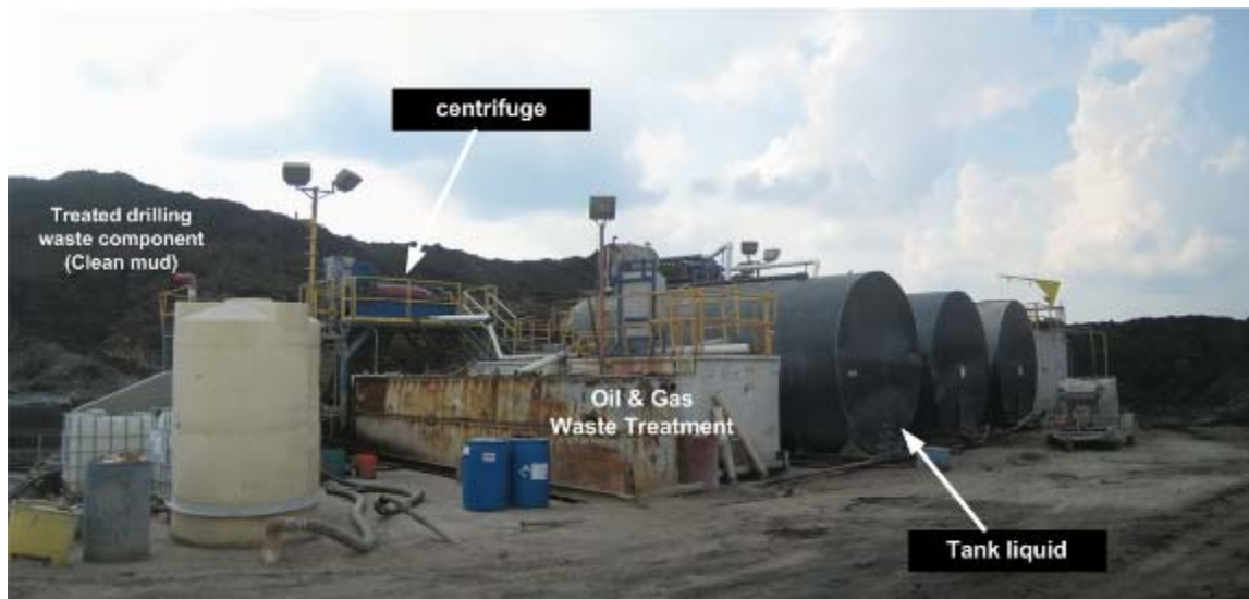
Figure 46. Oil and Gas Waste Treatment Equipment.
