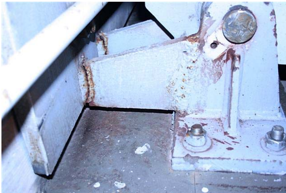
Figure 29. Photograph of Cracked Bearing Assembly.
