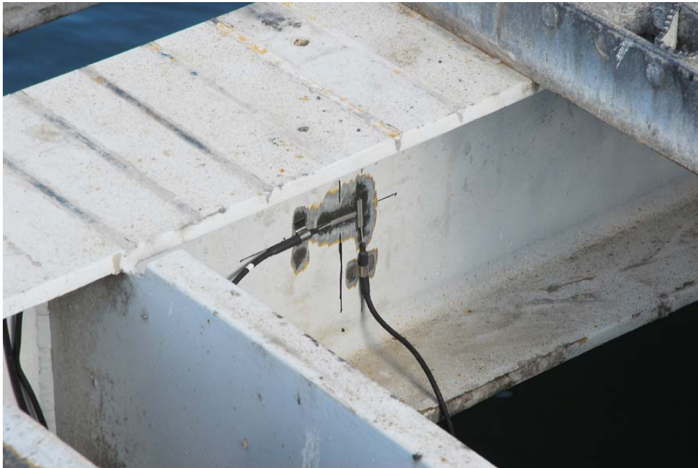
Figure 35. Photograph of Typical Sensor as Installed.
