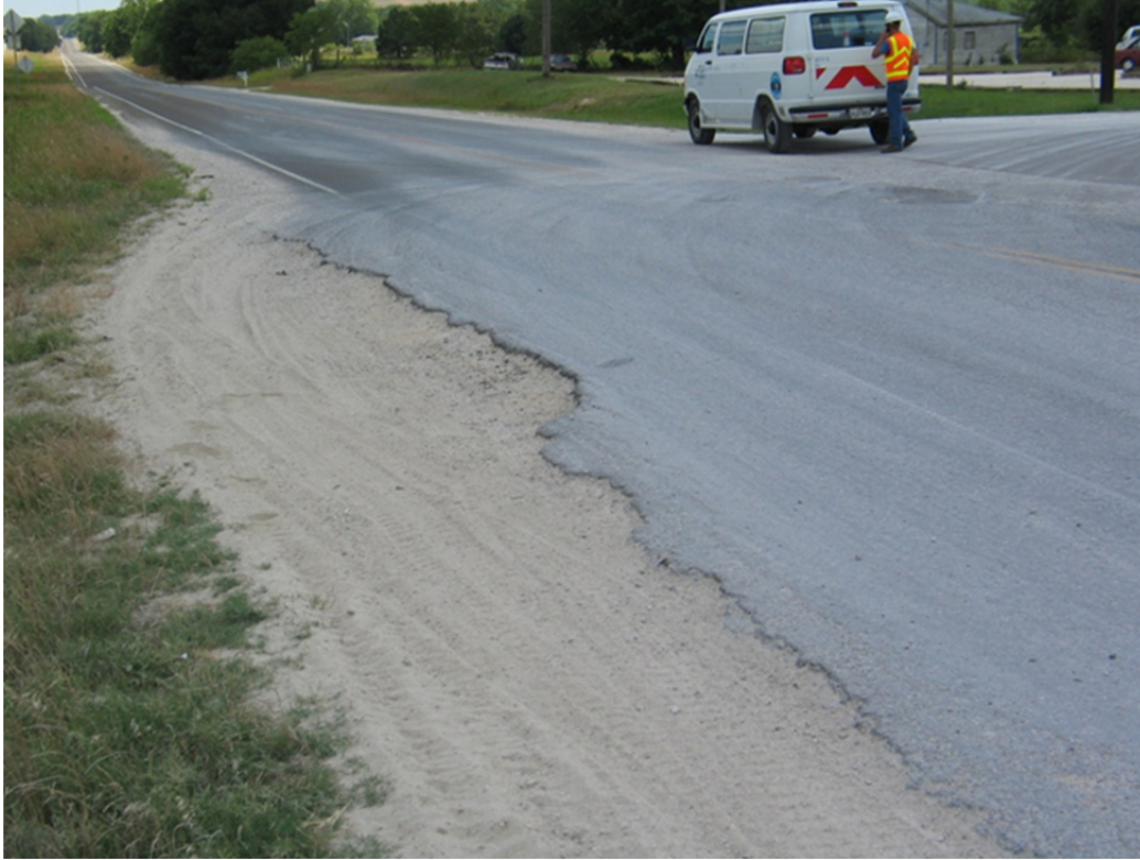
Figure 50. Tire Tracks on Unpaved Shoulder (IH 35W – Frontage, Fort Worth District).
