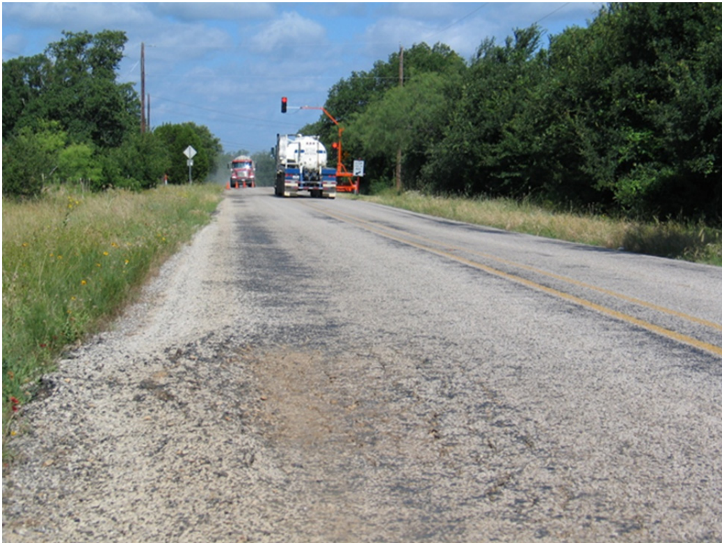
Figure 39. Failure, Flushing (FM 52, Fort Worth District).
