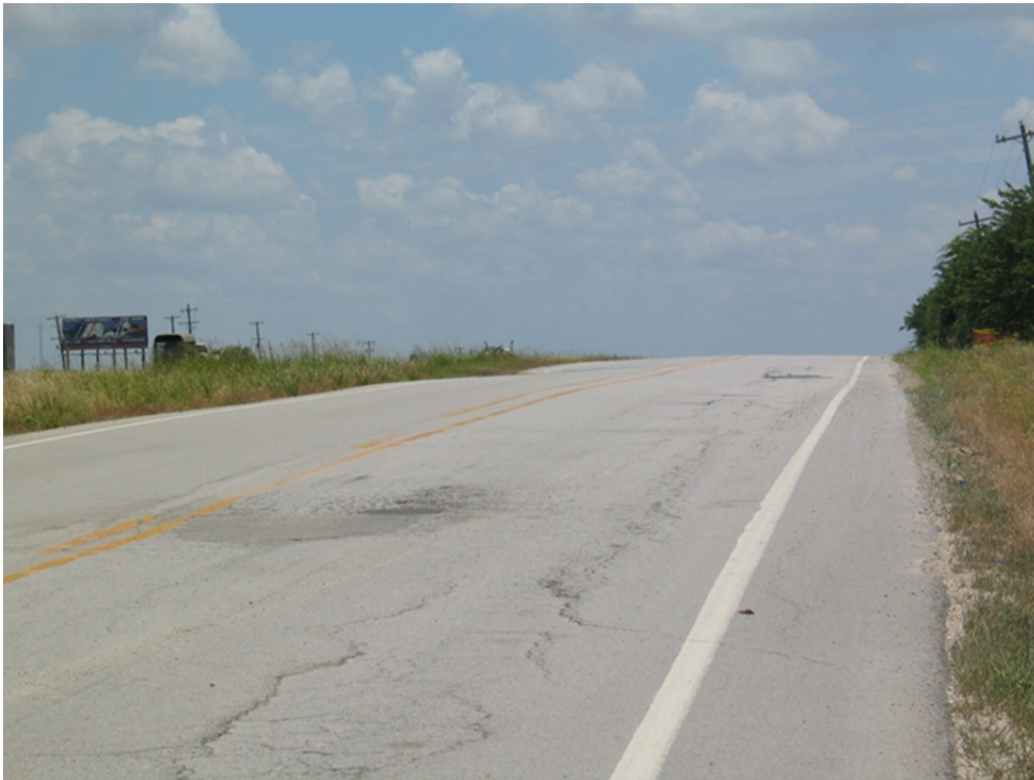
Figure 45. Alligator Cracking, Base Failure (IH 35W – Frontage, Fort Worth District).
