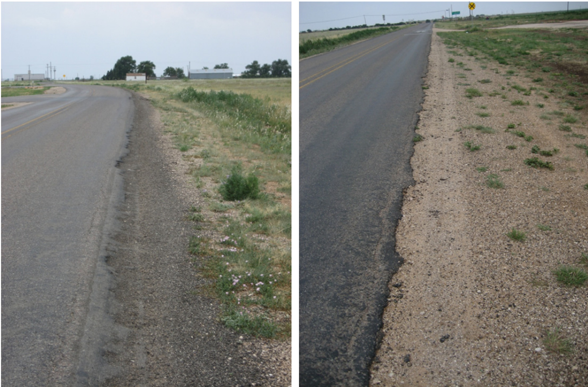
Figure 25. Edge Failure, Tire Tracks on Unpaved Shoulder (FM 2646, Lubbock District).
