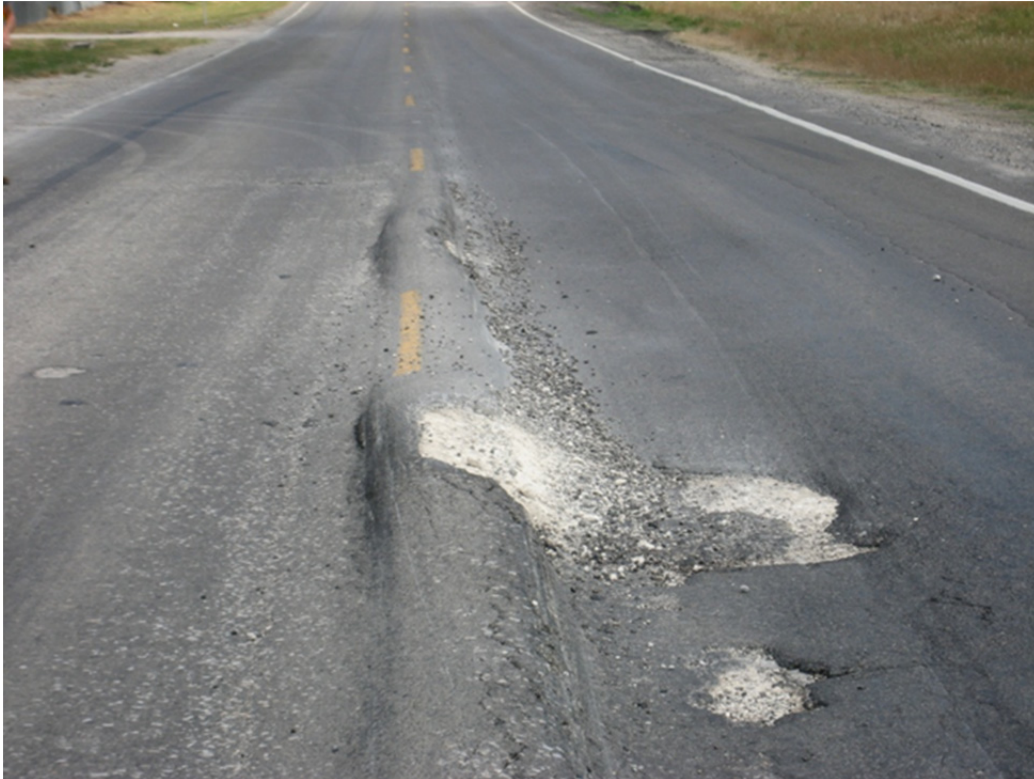
Figure 46. Pavement Shoving, Loss of Surface (IH 35W – Frontage, Fort Worth District).
