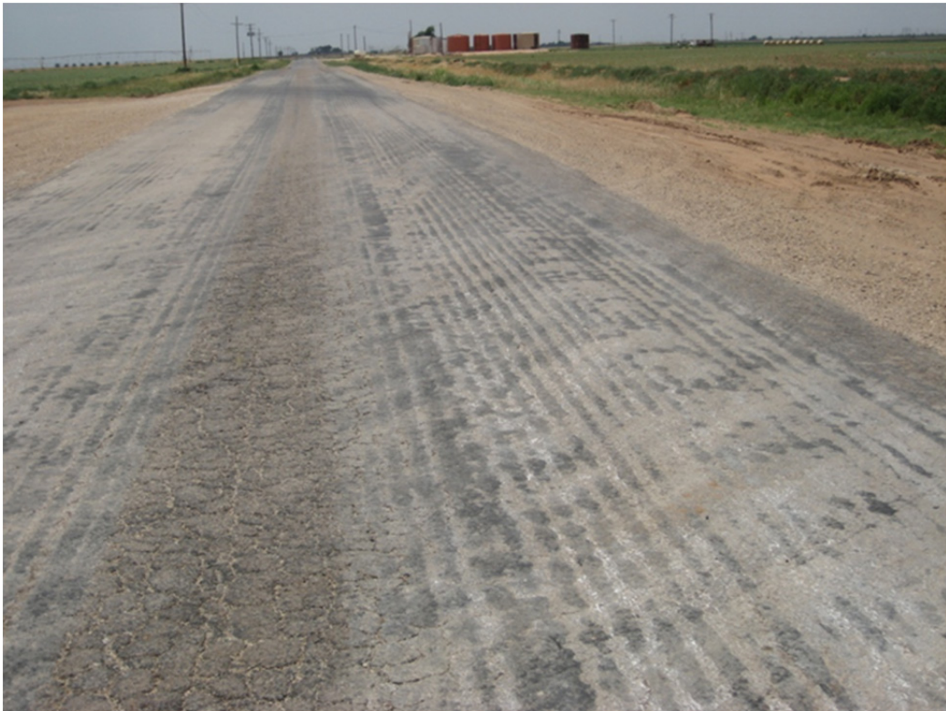
Figure 21. Pavement Failure, Surface Ripples (FM 1585, Lubbock District).
