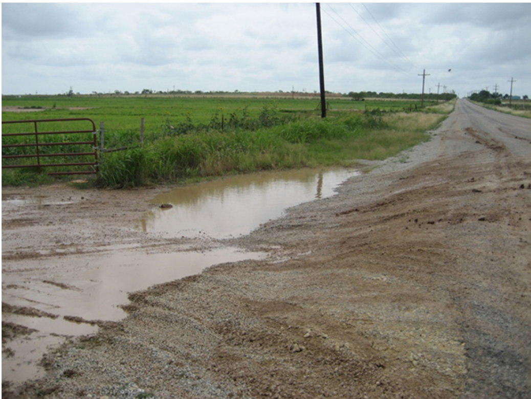
Figure 37. Drainage Problems (FM 1611, Abilene District).
