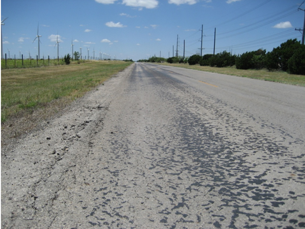
Figure 32. Failures, Alligator Cracks, Flushing (FM 89, Abilene District).
