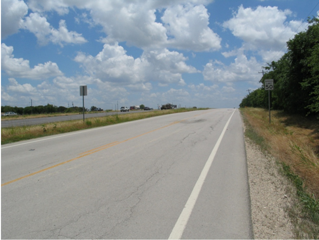
Figure 44. Alligator Cracking, Base Failure (IH 35W – Frontage, Fort Worth District).
