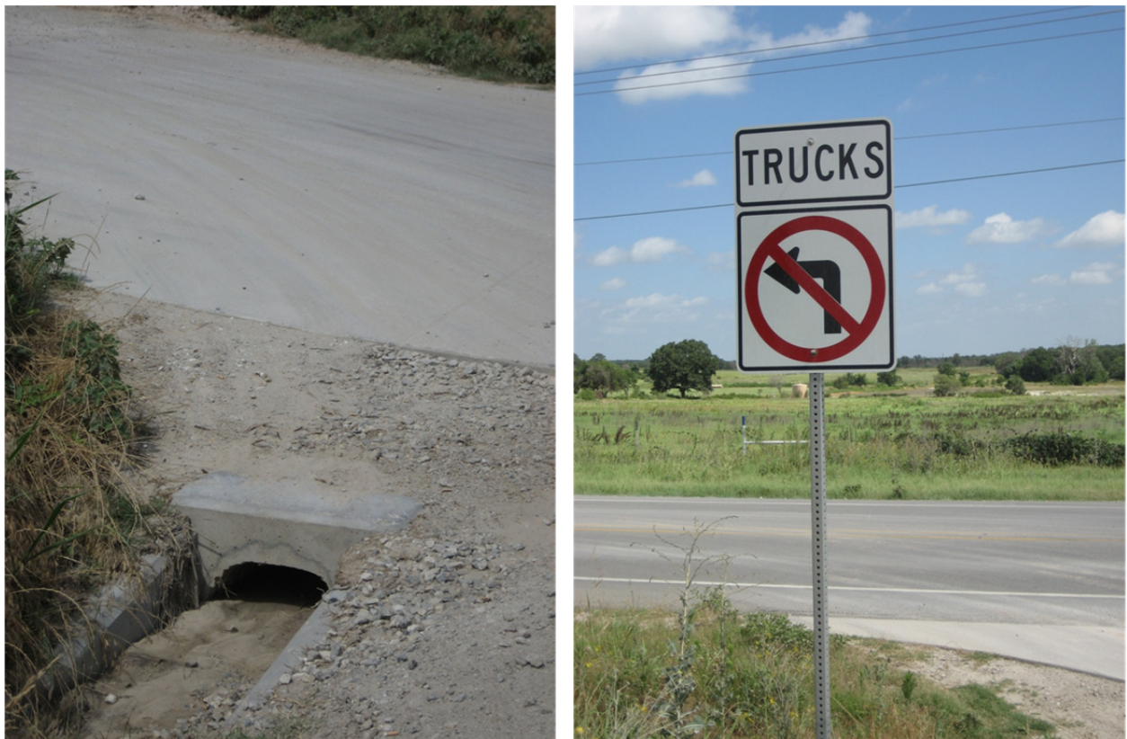
Figure 72. Tire Tracks on Driveway End Treatment and Illegal Left Turns (Fort Worth District).
