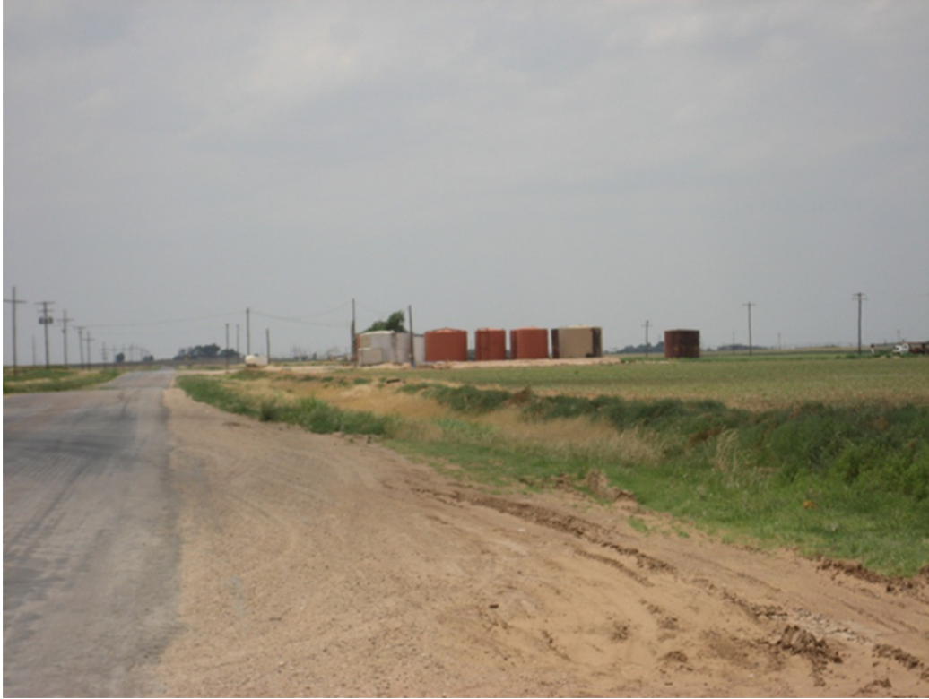
Figure 22. Shoulder Damage, Saltwater Disposal Facility (FM 1585, Lubbock District).
