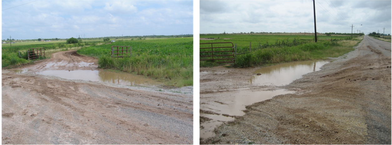
Figure 71. Drainage Problems and Mud Tracking (Abilene District).
