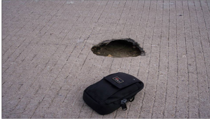
Figure 2.1. Large Void Generated by Clay Ball in Pavement in Central Texas.
