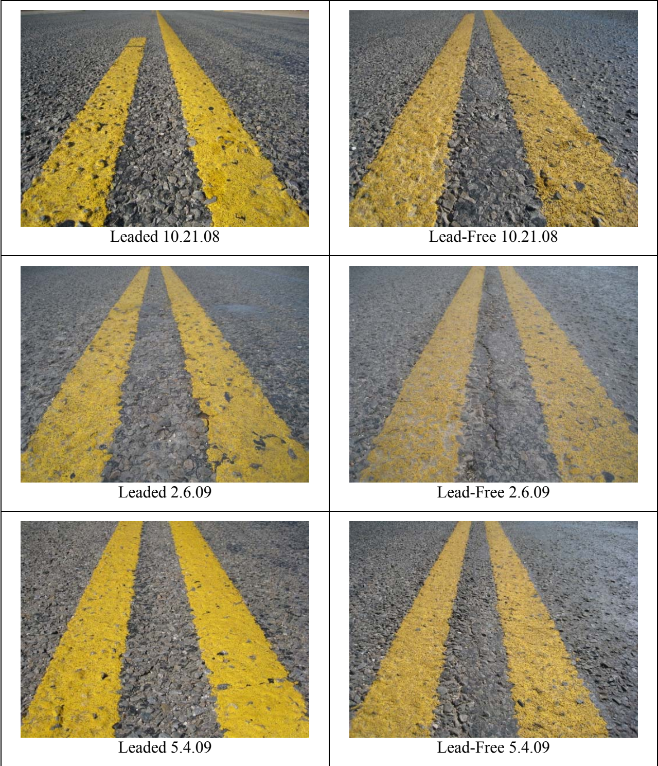
Figure F1. Photos of US 79 Leaded and Lead-Free Thermoplastic Markings over Time (continued).
