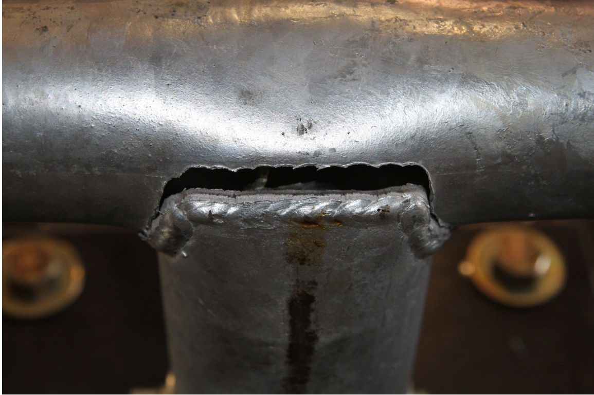
Figure 11.21. Deformation and Failure of U-Bracket Support.
