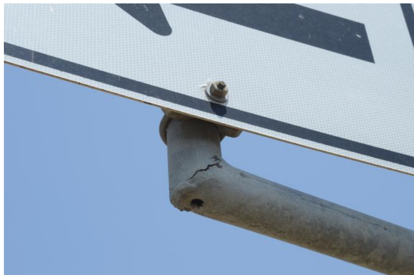
Figure 11.2. U-Bracket Weld Failure.
