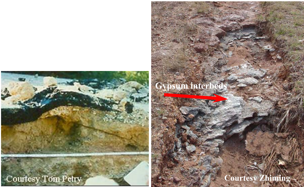
Figure 1.1. Heaves Observed at Joe Pool Lake due to Sulfate in the Soil (Left). Localized Sulfate Deposits Exposed in a Drainage Ditch (Right).
