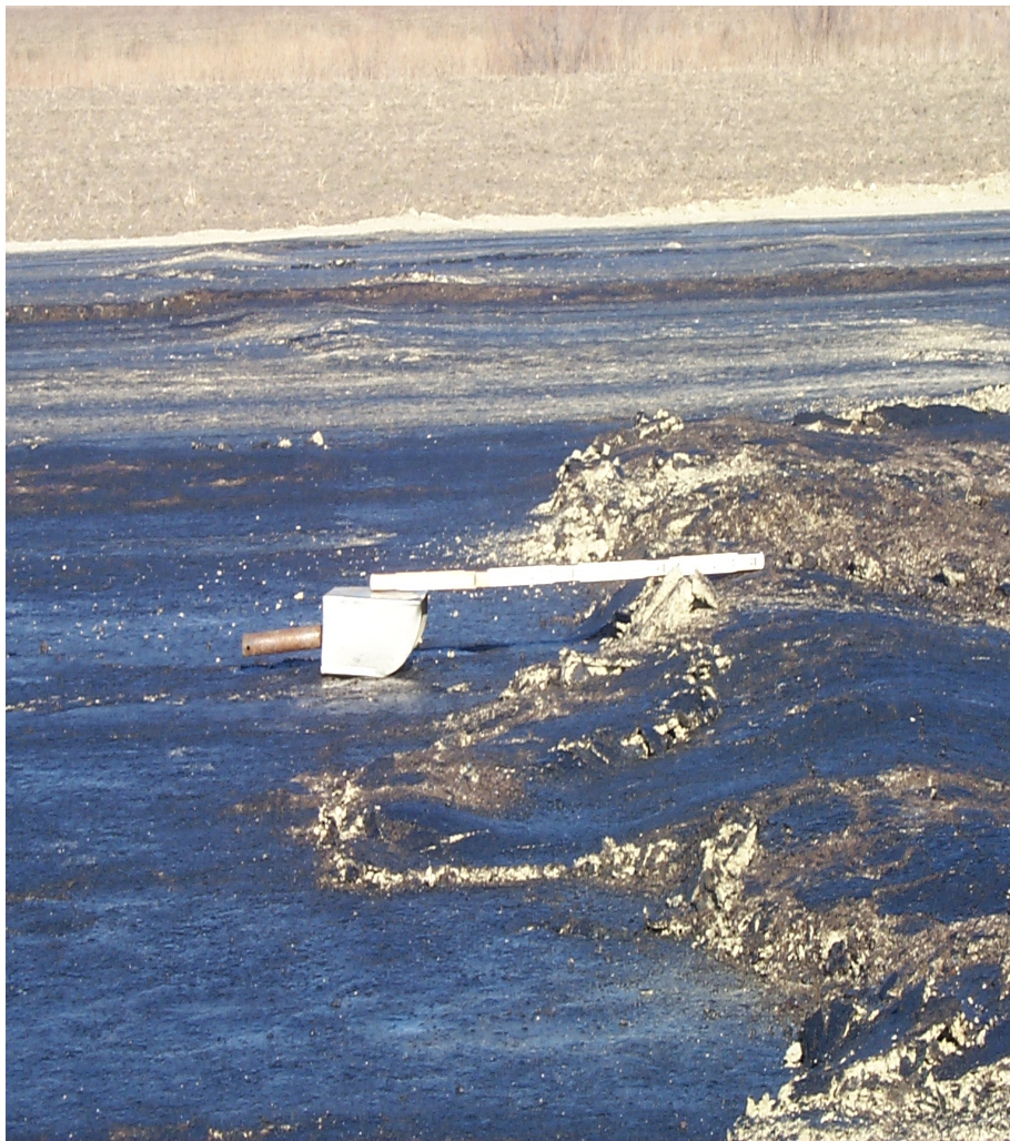
Figure 5a.1. US 67 in the Dallas District Showing Distress due to Sulfate Heave.
