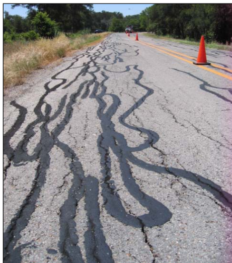
Figure 4.7. Longitudinal Cracking on FM 112.
