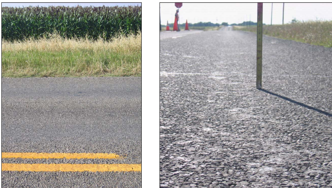
Figure 3.1. Rutting on FM 487.
