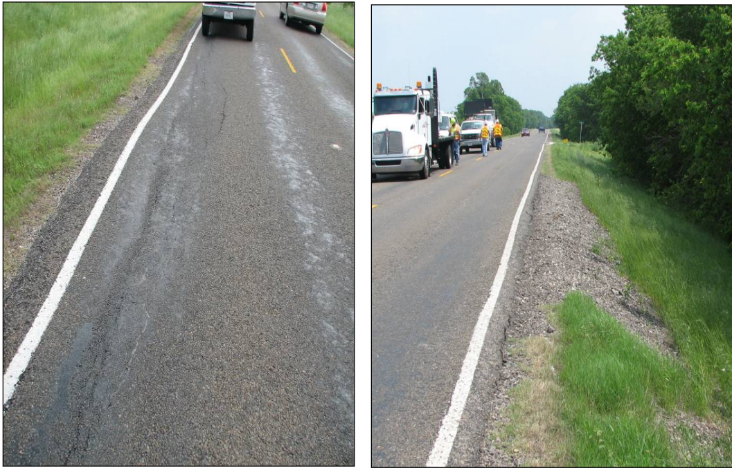
Figure 7.1. Typical Edge Failure on FM 148.
