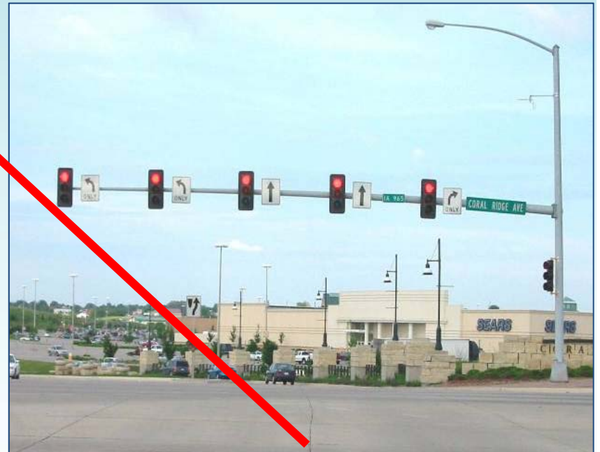
Example - 12-inch heads, one signal head per lane, back plates
