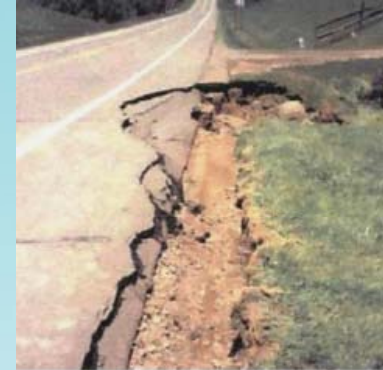
Deterioration of pavement edge and shoulder due to poor drainage.
