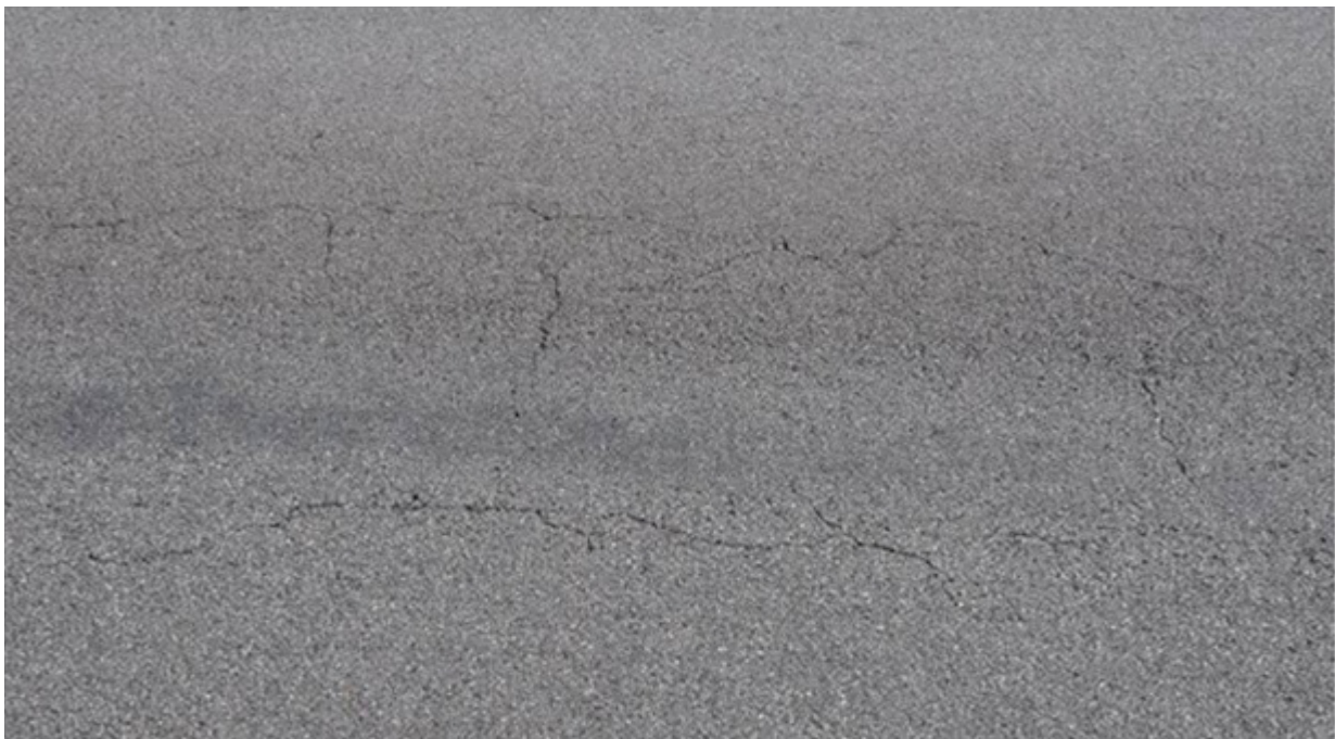
Figure 6-2. Example of Pre-Existing Cracks on Control Section 01 (ATL).
