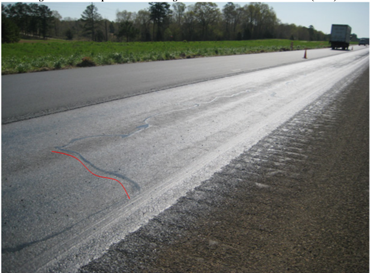
Figure 6-4. Example of Pre-Existing Cracks on Control Section 02 (ATL).
