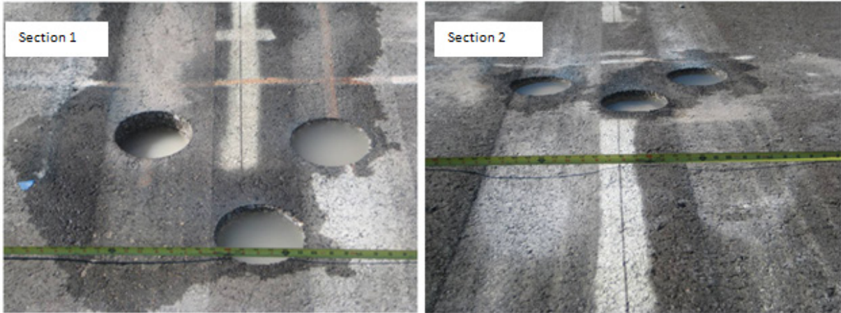
Figure 5-3. Surface Rutting on Sections 1 (Control) and 2 (Modified).
