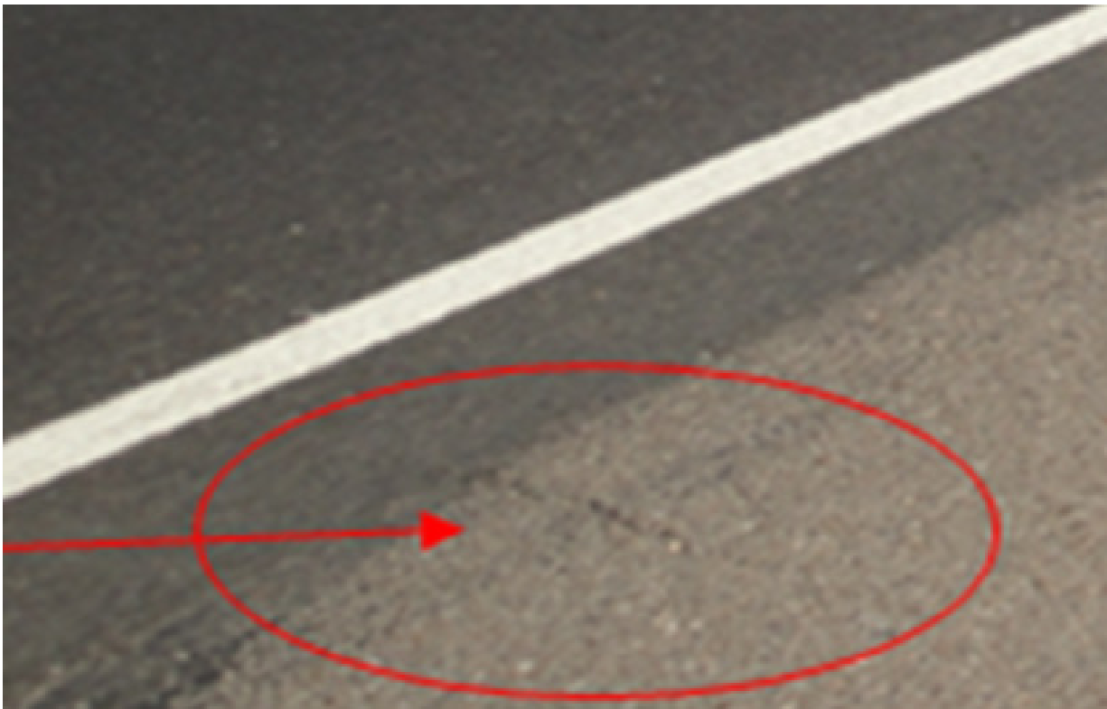
Figure 6-14. Example of Cracking on Loop 20 prior to 2 inch HMA Overlay. Construction Monitoring – HMA Placement
