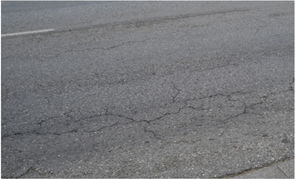
Figure 6-13. Example of Cracking on Spur 400 prior to 2 inch HMA Overlay.
