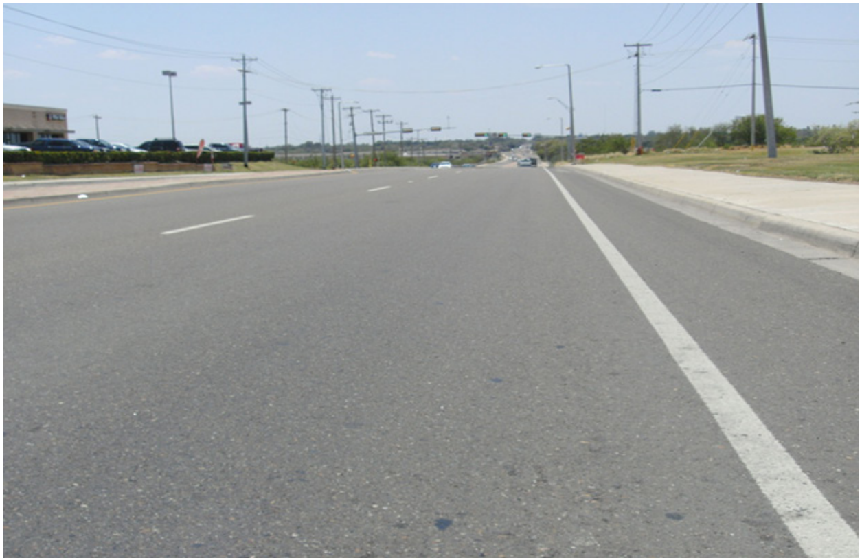
Figure 6-18. Field Performance – Spur 400 (Oct 2012) – No Distresses (LRD).
