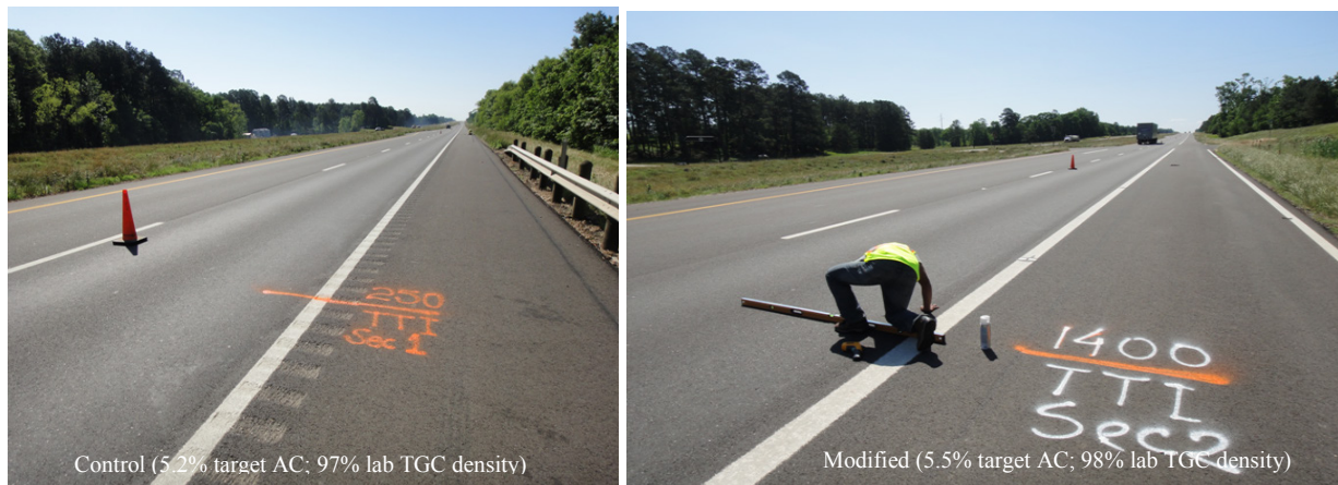
Figure G-2. View of the Test Sections – No Visible Surface Rutting or Cracking – ATL. (After 2 Years; April 2012).
