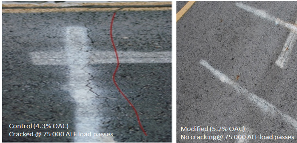
Figure 5-6. Reflective Cracking Comparison of Section 4 (Control, LTE = 50 Percent) and Section 6 (Modified, LTE = 50 Percent) after 75,000 ALF Load Passes.
