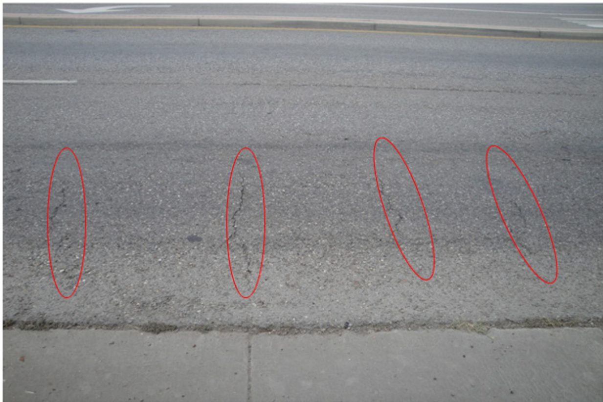
Figure 6-12. Example of Cracking on US 59 prior to 2 inch HMA Overlay.
