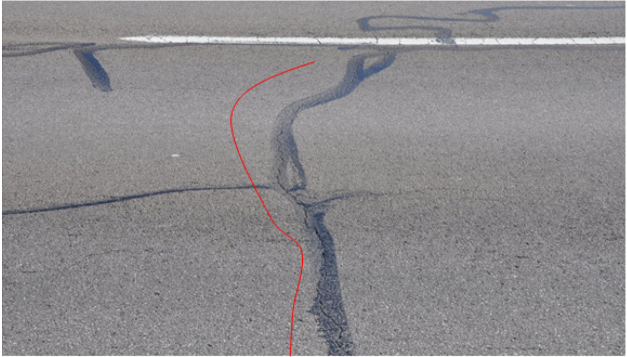
Figure 6-3. Example of Pre-Existing Cracks on the Modified Section (ATL).
