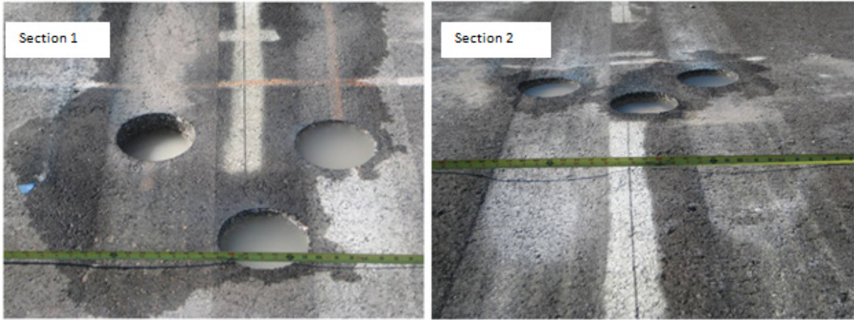
Figure 5-2. Surface Rutting on Sections 1 (Control) and 2 (Modified).
