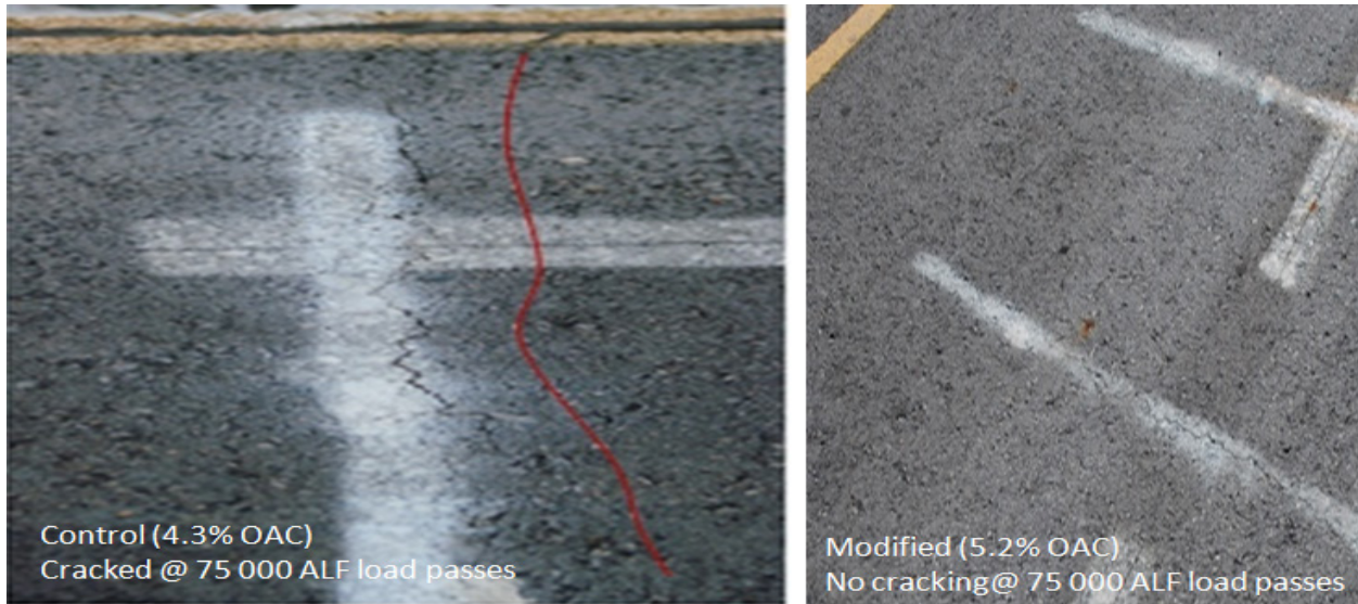
Figure 5-5. Reflective Cracking Comparison of Section 4 (Control, LTE = 50 Percent) and Section 6 (Modified, LTE = 50 Percent) after 75,000 ALF Load Passes.
