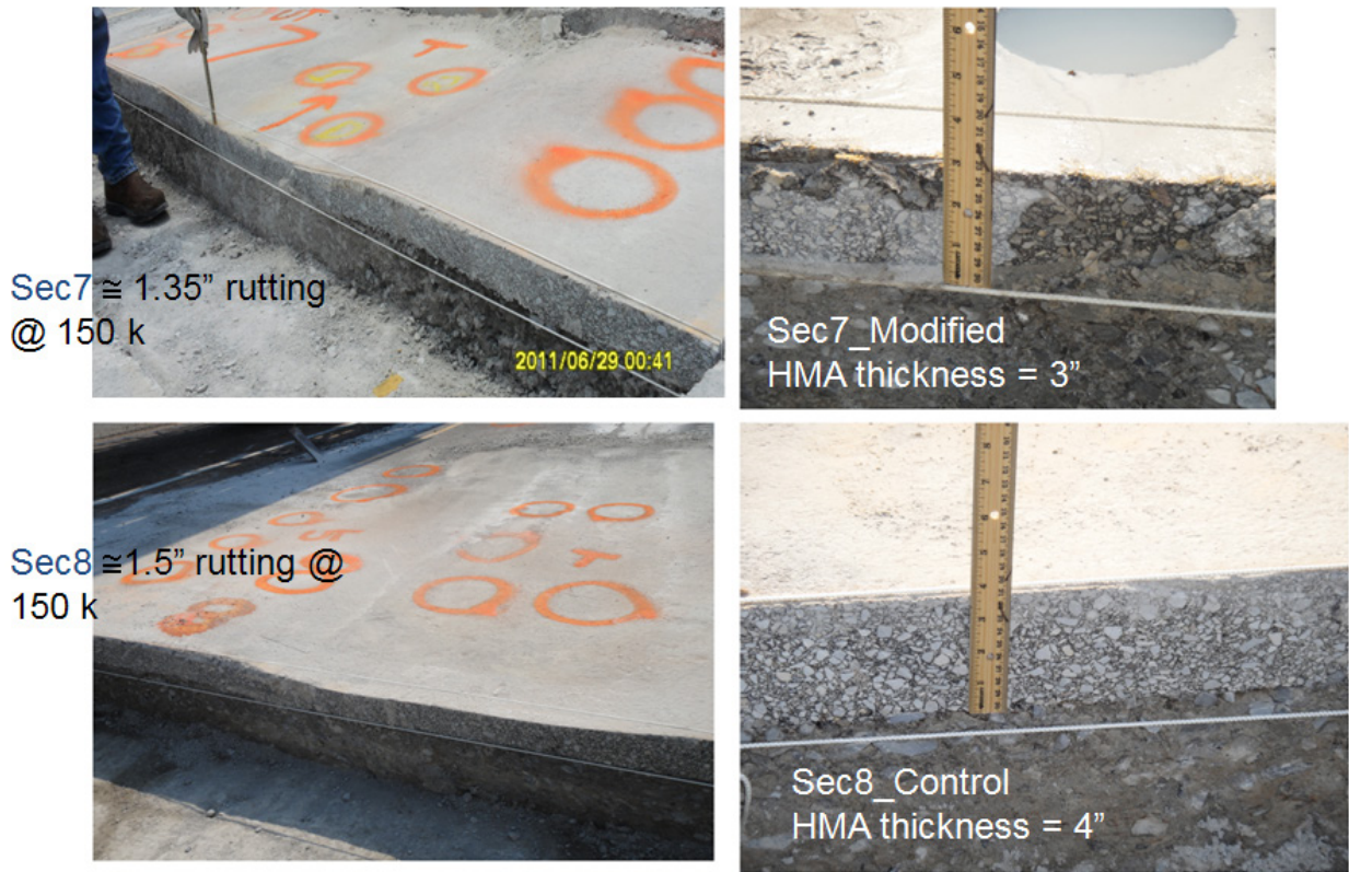
Figure 5-8. Base-Subgrade-Related Rut Failure on the Fatigue Crack Sections 7 and 8.
