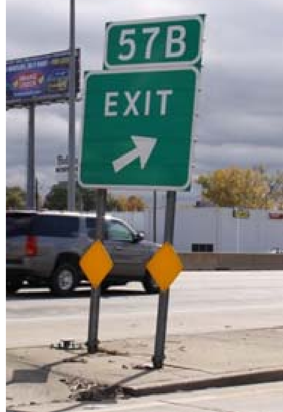
Figure 24. Reflective Object Markers on Sign Posts.
