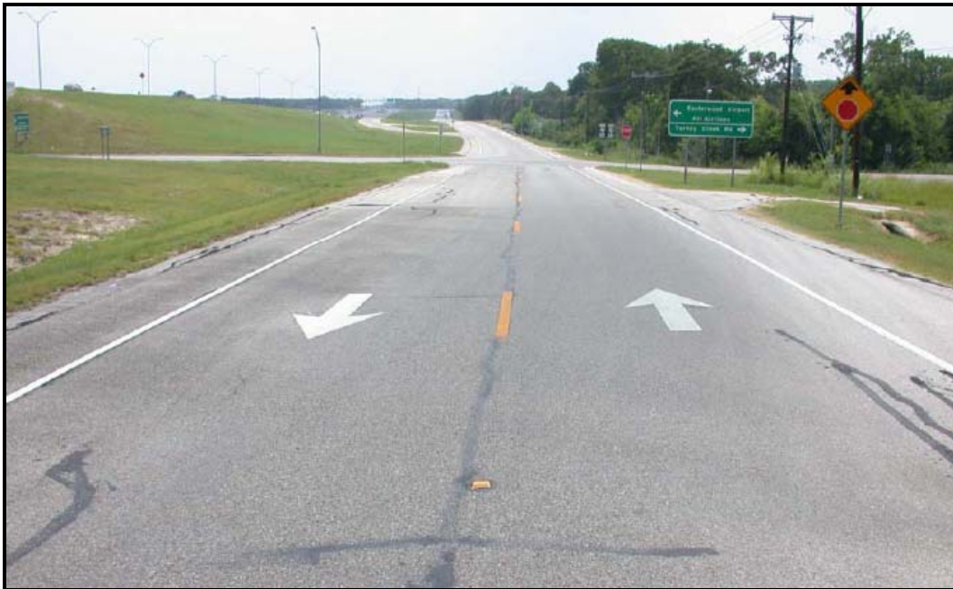
Figure 17. View of Frontage Road Lane Use Guidance after Arrow Pavement Marking Installation. (3)
