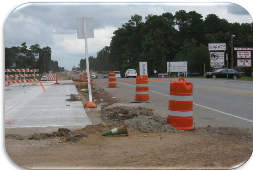
Figure 26. Driver's View from a Passenger Car on a Minor-Road Approach in a Work Zone.
