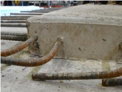
(a) Cracking between Stage I and II
