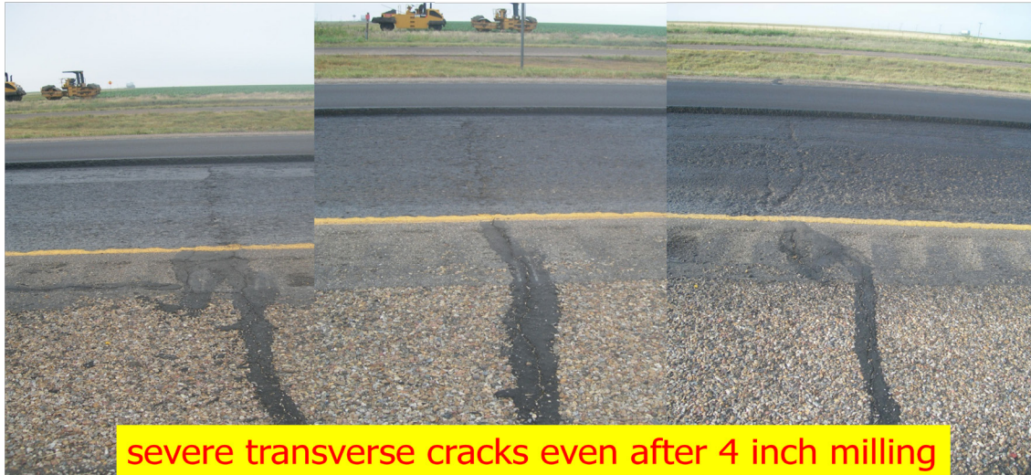
Figure 3. Existing Pavement Conditions of IH40 after Milling.
