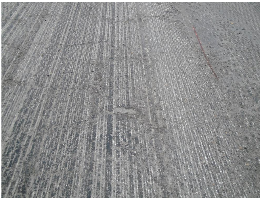
Figure 5. Observed Cracking after 3 inch Milling on SH359.
