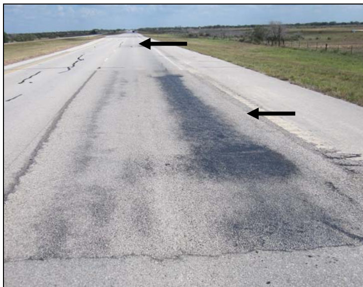
Figure 55. Patching on US 77.
