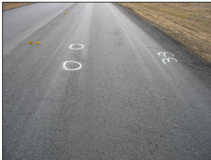
Figure 80. Visually Observed Segregation on FM 2440 after Construction.
