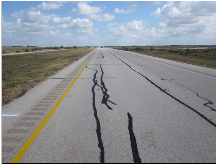
Figure 51. US 77 Section after Five Years of Service.
