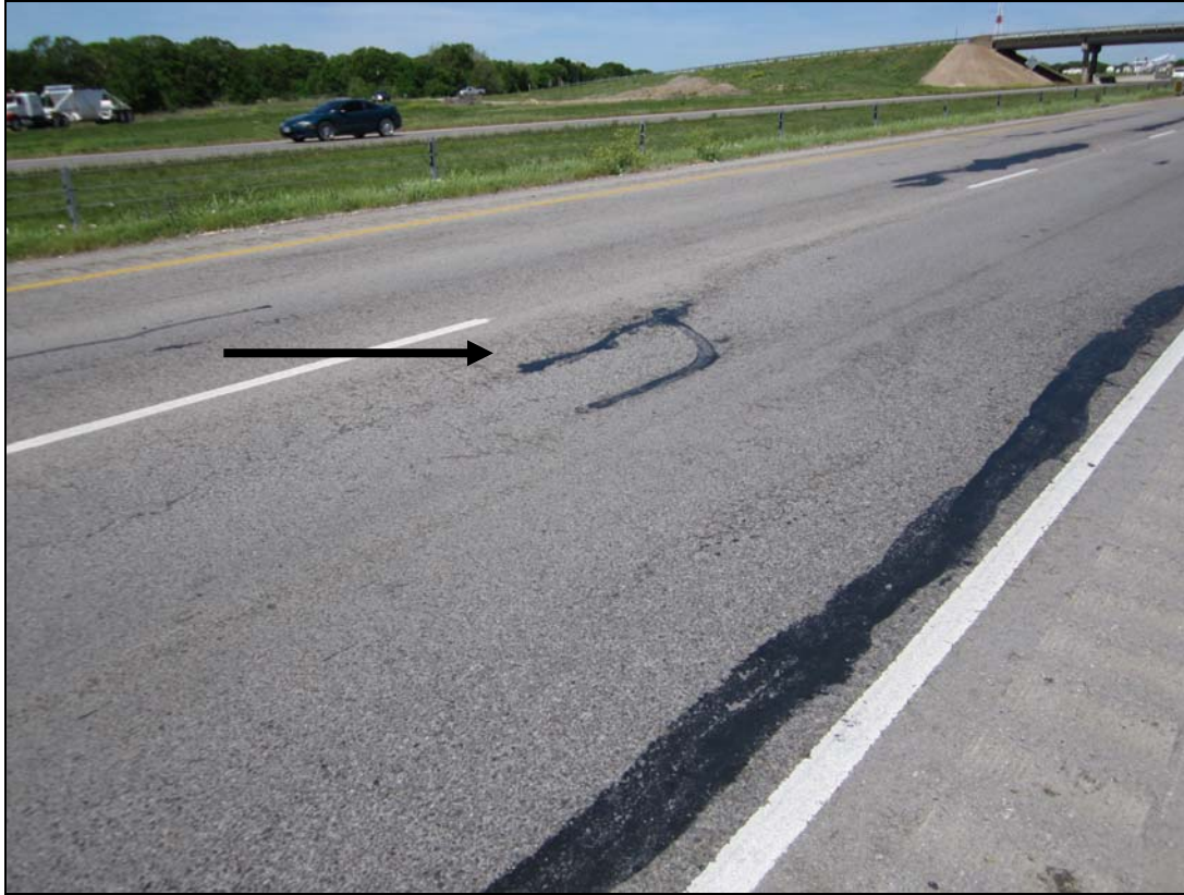
Figure 111. Raveling and Cracking Failures in Segregated Zones on IH 35W.
