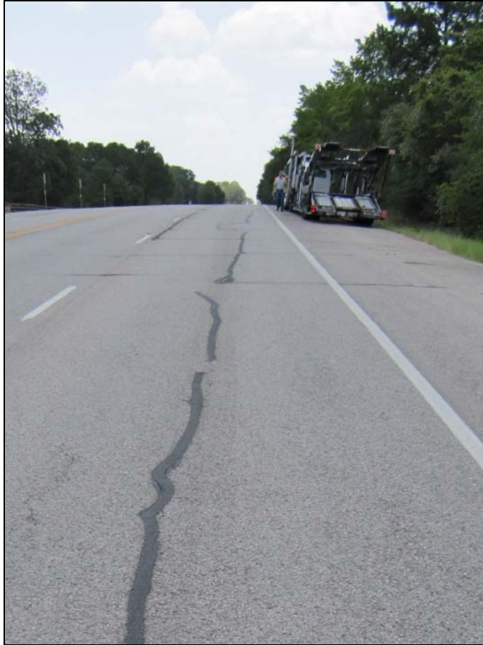
Figure 43. Transverse and Longitudinal Cracking on BU 290.
