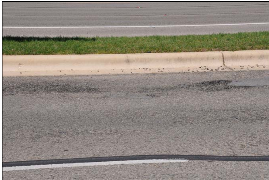
Figure 107. Severe Raveling on A.W. Grimes.
