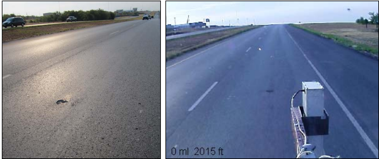
Figure 35. Localized Distress on US 81.
