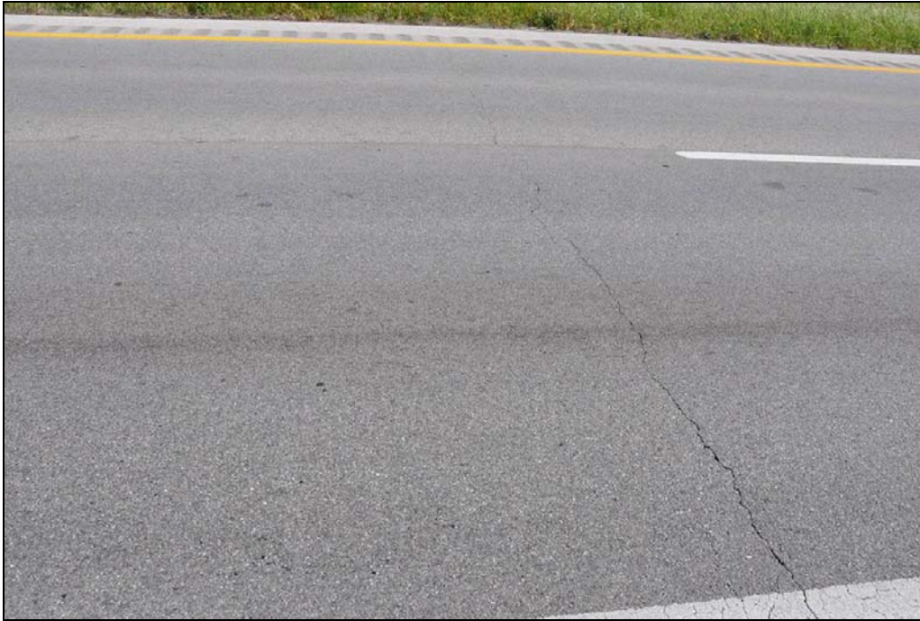
Figure 8. Example Transverse Cracking on IH 10 after Four Years of Service.
