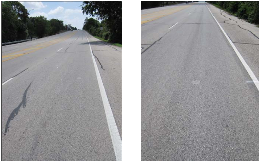
Figure 45. Thermally Segregated Locations on BU 290 after Seven Years of Service.
