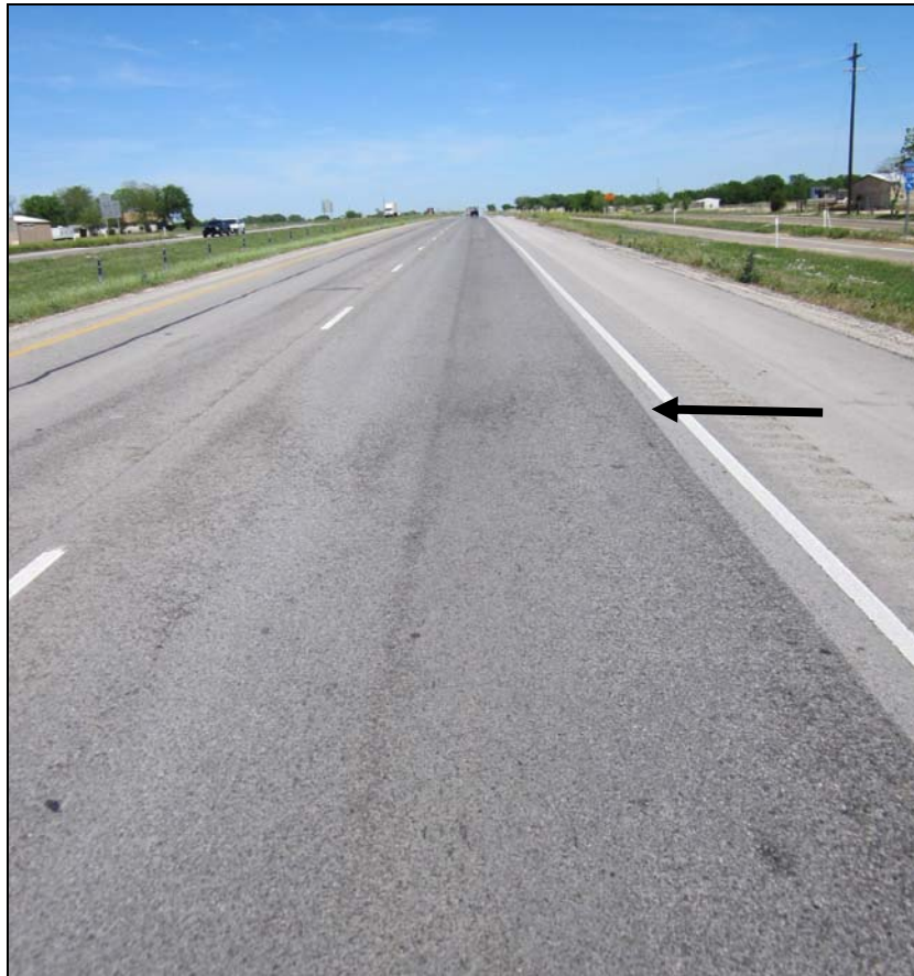
Figure 110. Zone of Cyclic Segregation on IH 35W.
