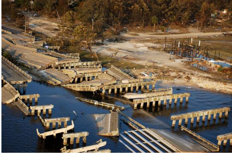
Figure 1. Highway 90 Bridge Damaged during Hurricane Katrina The bridge was located on US-90 in Biloxi and Gulfport, Mississippi Gulf Coast (from Gulf Coast Information System, 2006 ).
