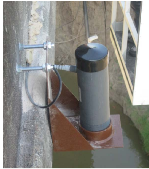
Figure D-18. Installed Water Stage Sensor.
