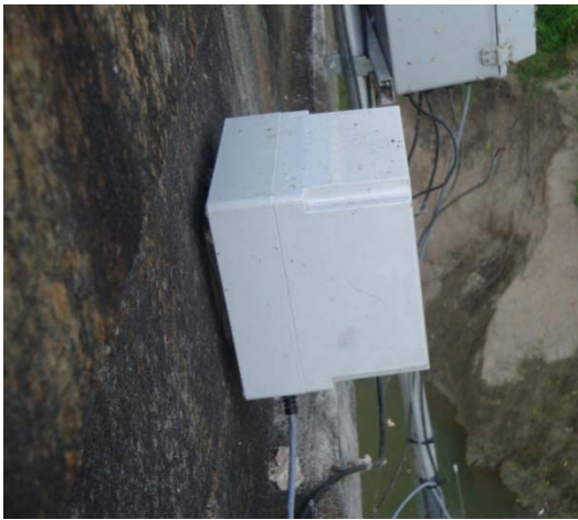
Figure D-13. Single-Axis Tiltmeter 1 on the Deck Adjacent to Master Station at Pier SB2.
