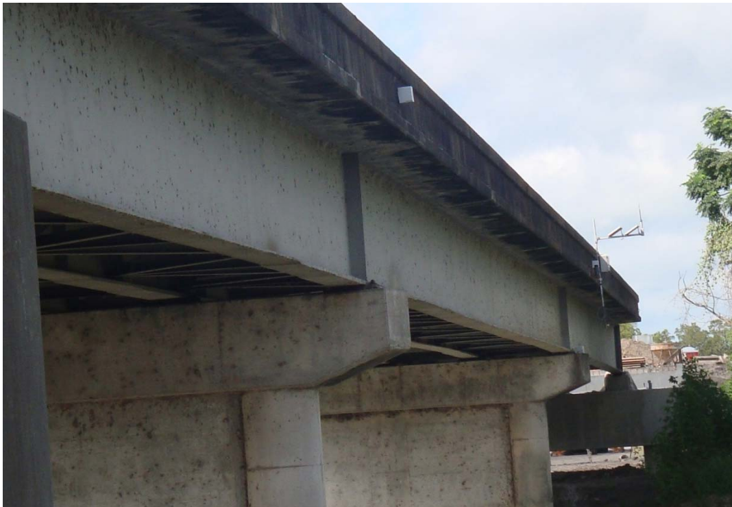
Figure D-16. Bridge Scour Monitoring System (View from North Side of the Bridge).
