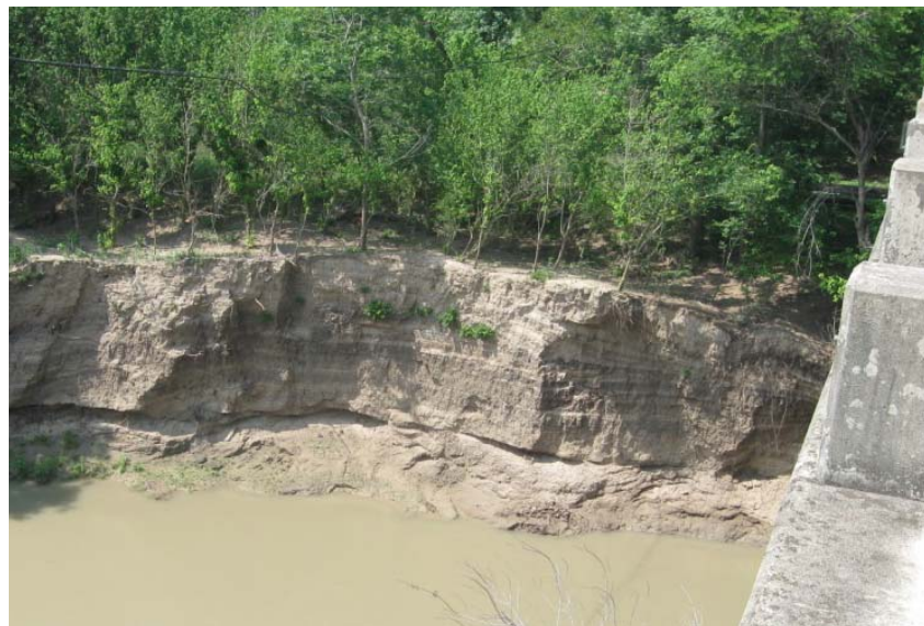
Figure E-10. Southern Bank of San Antonio River (Downstream of the Bridge).
