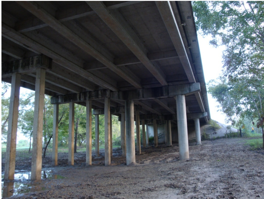
Figure E-6. Eastern Approach Spans of SH80 over San Antonio River Bridge.
