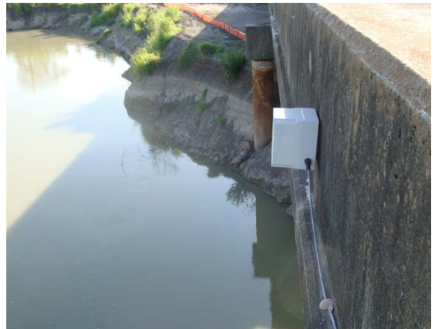
Figure D-14. Single-Axis Tiltmeter 2 on the Deck at Pier SB1.
