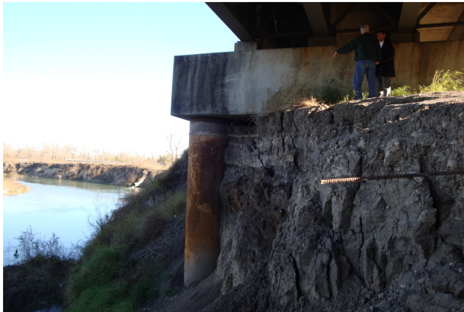
Figure 5-5. Drill Shaft on Northeast Side (SB0) of US59 over Guadalupe River Bridge in 2009.
