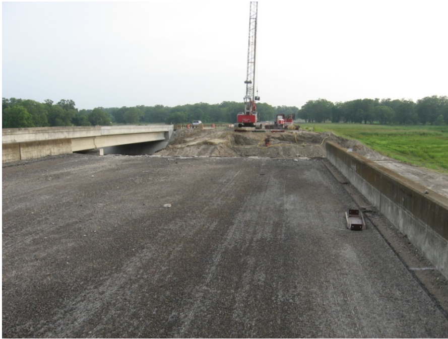
Figure D-40. Construction on the Extension of the Southbound Lane of US59 over Guadalupe River Bridge.
