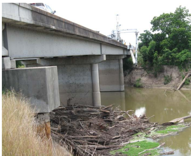
Figure D-7. Working on a Snooper Truck (SB1 is front pier with debris).
