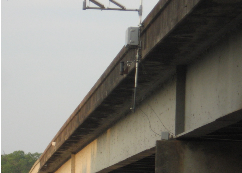
Figure D-15. Bridge Scour Monitoring System (View from South Side of the Bridge).
