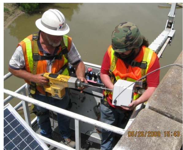
Figure D-8. Drilling a Hole in the Tiltmeter Enclosure to Install the Bolt.
