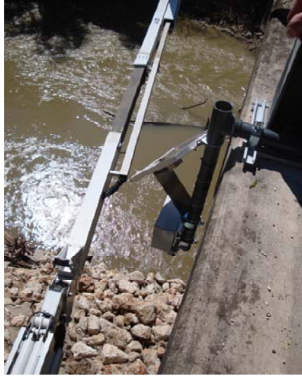
Figure 6-15. Solar Panel for the Accelerometer on the Cap Beam of Pier P1.
