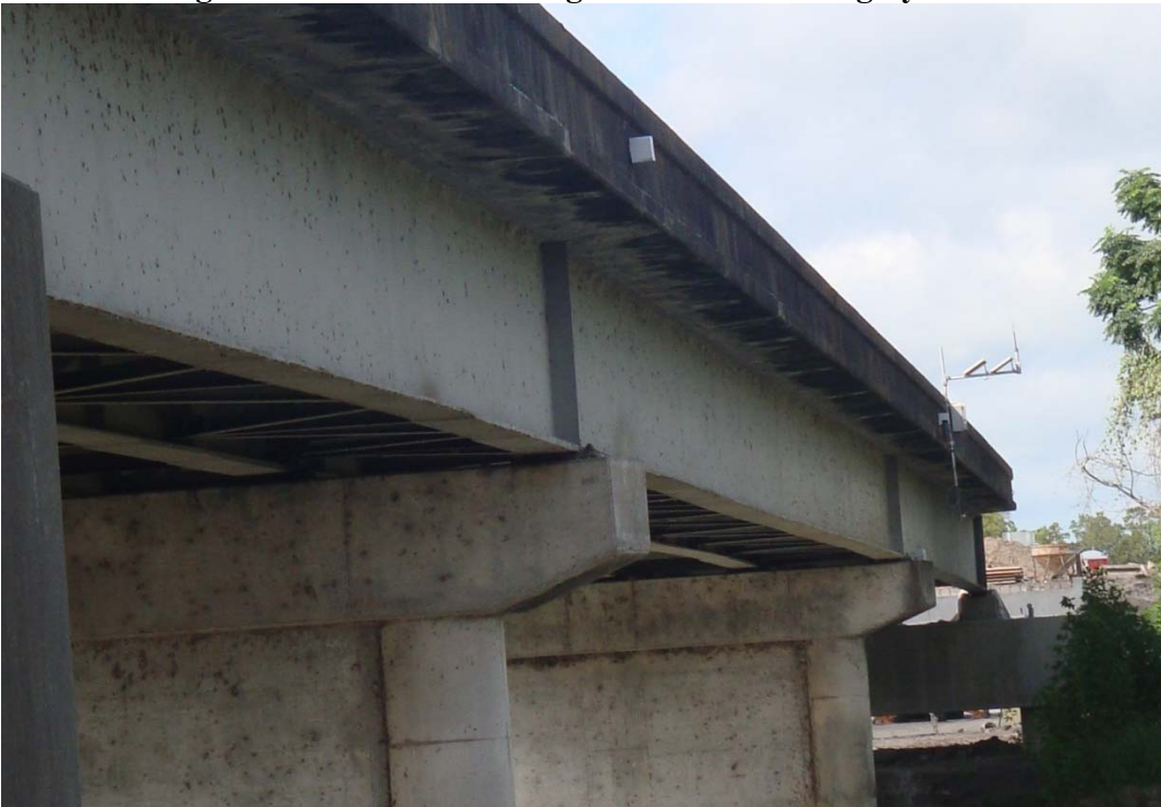
Figure 5-29. Modified Bridge Scour Monitoring System.
