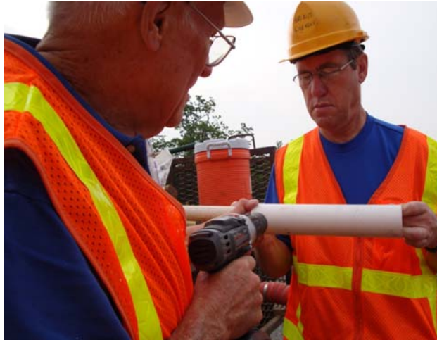
Figure 5-15. PVC Pipe as an Extension of Float-Out Device.
