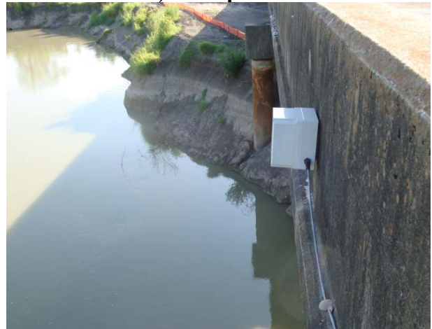
Figure 5-27. Single-Axis Tiltmeter (Tiltmeter2) on the Deck (Near Pier SB1).
