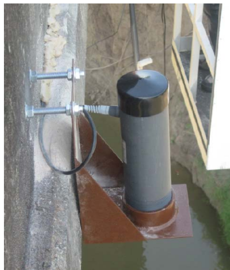
Figure 5-10. Installed Water Stage Sensor.
