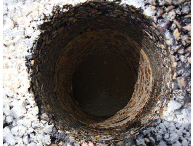
Figure D-20. Close-Up of the Drilled Hole in the Deck.
