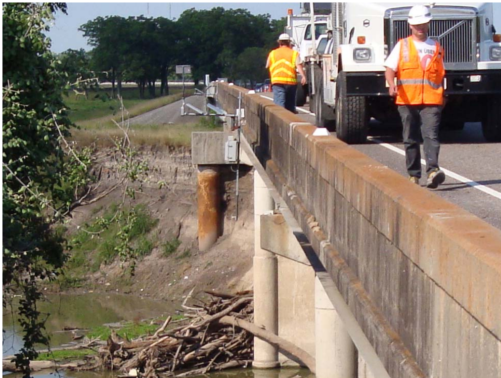
Figure 5-24. Initial Bridge Scour Monitoring System.
