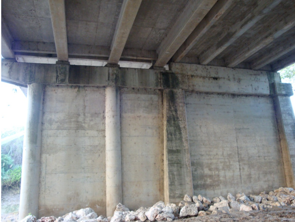
Figure E-5. Compound Concrete Web-Wall Pier P1 on the Bridge Main Span.
