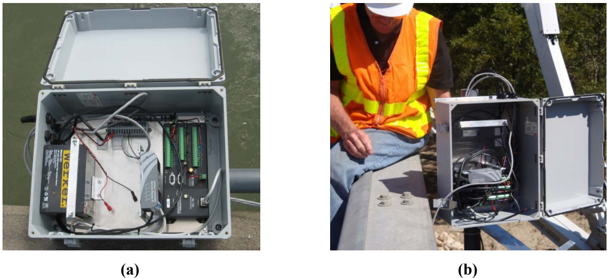
Figure E-12. Master Station on SH80 over San Antonio Bridge: (a) During Installation and (b) After Installation.
