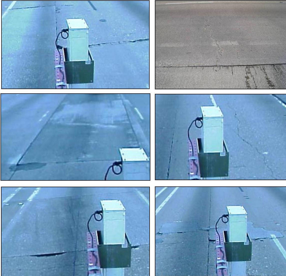
Figure 27. Surface Condition of Sampled Section on IH 635.
