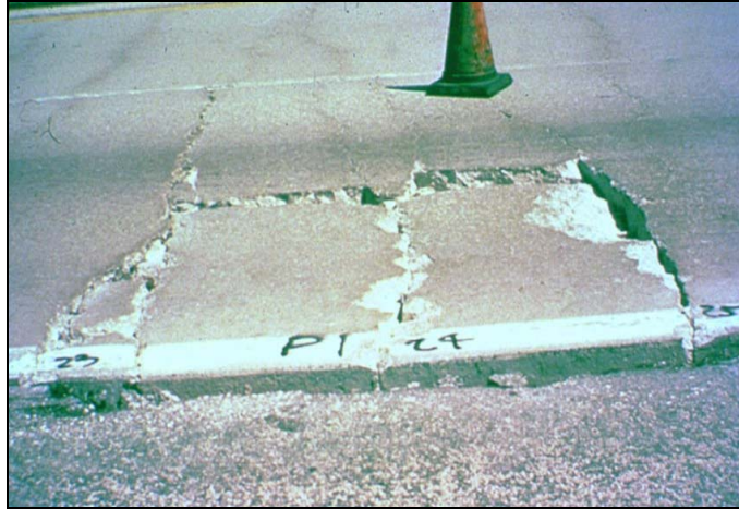
Figure 1. Effects of Erosion on CRC Pavement Performance.
