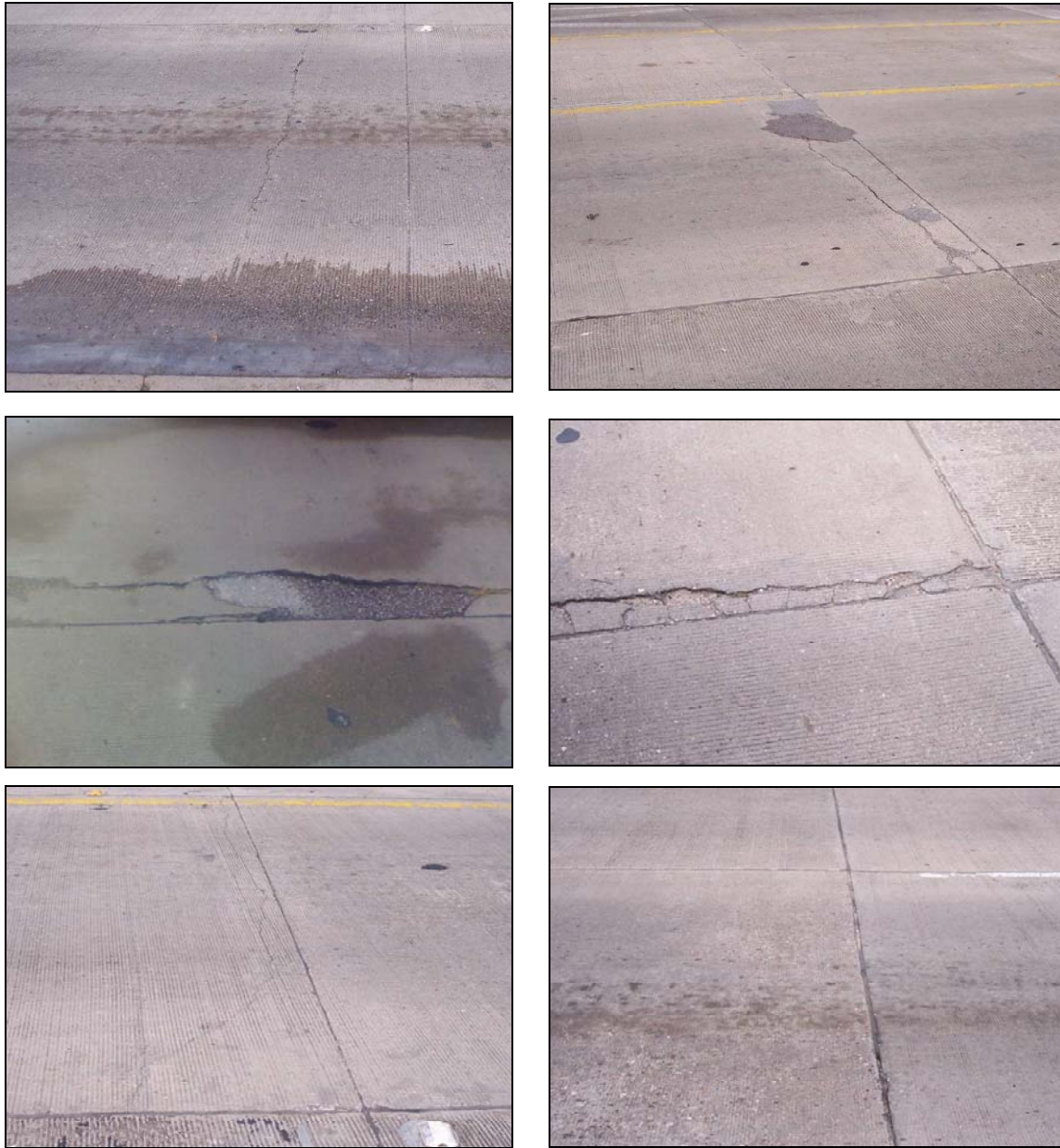
Figure 17. Surface Conditions of Sampled Section on FM 364.
