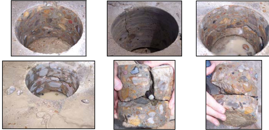
Figure 26. Interface and PCC Layer Condition of Section on IH 10.
