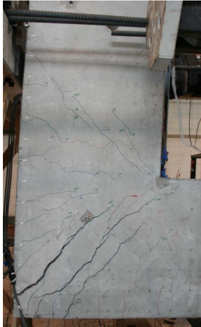
(a) Photograph of crack pattern at incipient failure near end of experiment.
