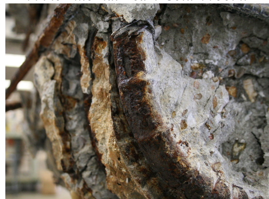
(f) Corrosion of Longitudinal Steel at the Exterior Knee-Joint
