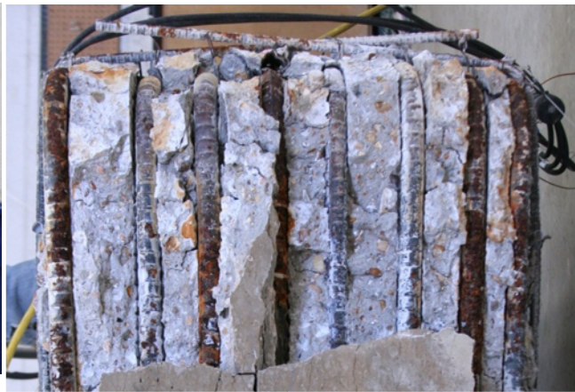
(f) Exterior face of the beam-column joint showing bulging of the U-bars, laterally displaced longitudinal steel, and reinforcing steel corrosion
