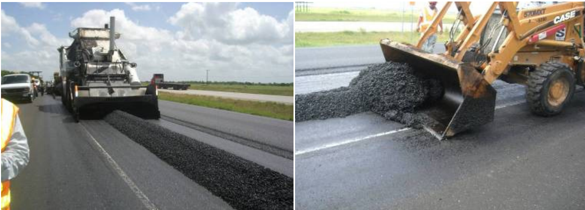
Figure 93. Windrow Pick-Up Process on US 59 in the Yoakum District with Cold Lumps Forming at the End of the Windrow.
