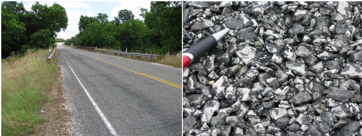
Figure 71. Raveling Distress on US 90 in Houston.
