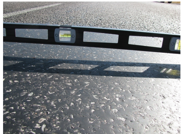
b) Detailed View of Bleeding and Rutting
