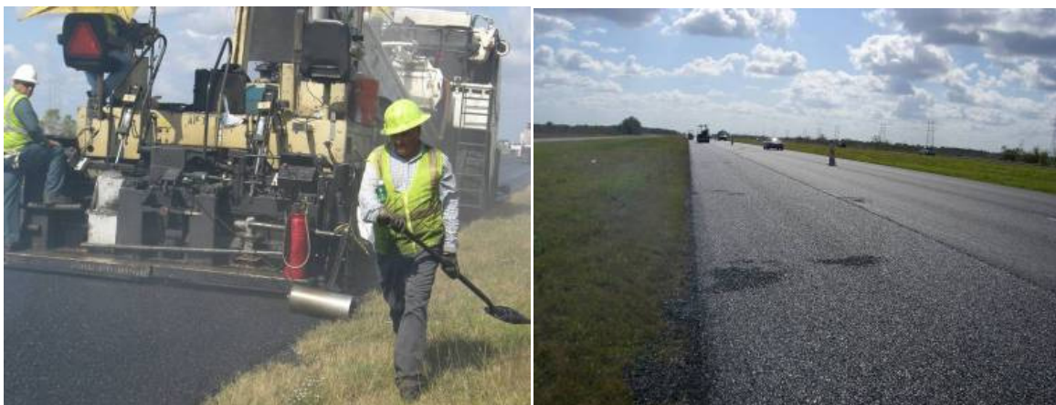
Figure 92. MTV Paving Operation (left photo) and Areas in the Mat Where Cold Chunks Required Removal and Patching (right photo) on US 288 in the Houston District.
