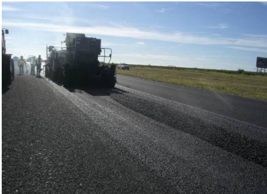
Figure 89. Application of PFC on Tacked, Newly Seal Coated Surface of IH 10 in Odessa District.
