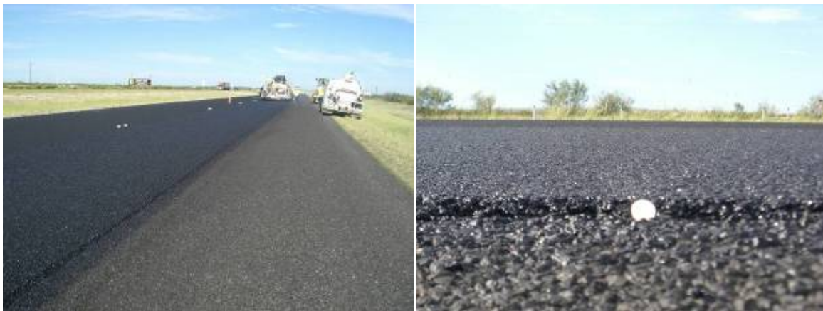
Figure 84. PFCs on Rural Interstates (Odessa District IH 10, AR Underseal Followed by AR-PFC).
