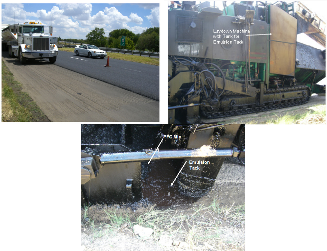
Figure 90. Laydown Machine with Tank for Applying Tack on IH-30 in the Paris District.
