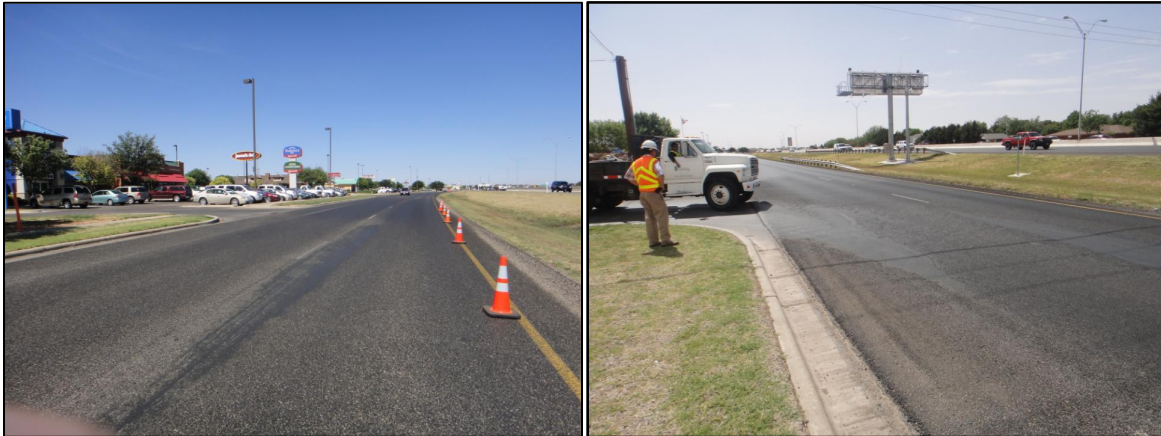
Figure 74. Raveling Distress on SL 289 in Lubbock.
