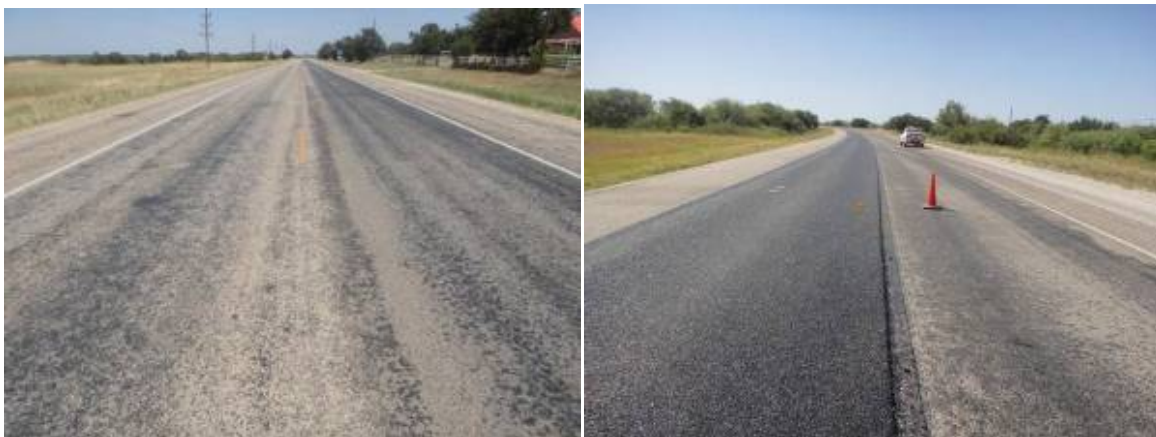
Figure 85. US 183 Brownwood District (PFC Used to Remediate Bleeding Surface Treatment).
