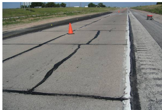
Poor Condition Section
