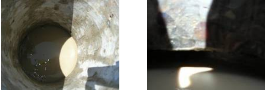
a) Void and Erosion under the Concrete Slab of Poor Condition Section
