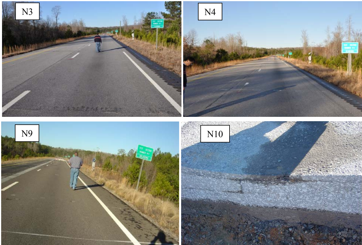
Figure 4-23. Sections without Fatigue Cracking: N3, N4, N9, and N10.
