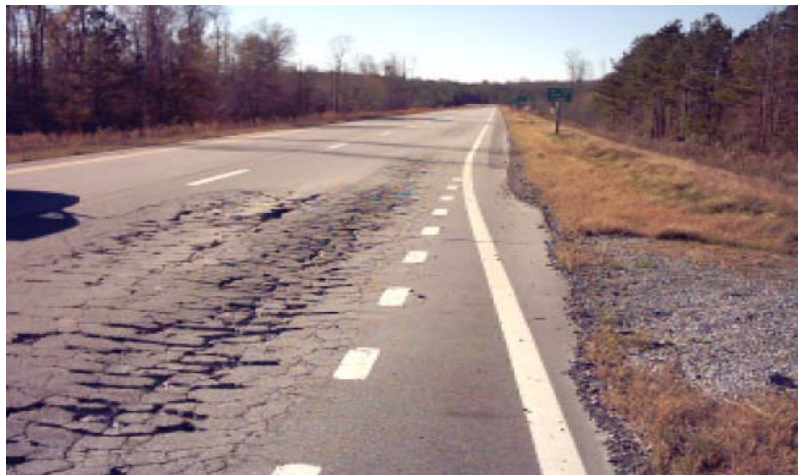
Figure 4-28. Observed Fatigue Cracking at Section N1 (NCAT 2005).
