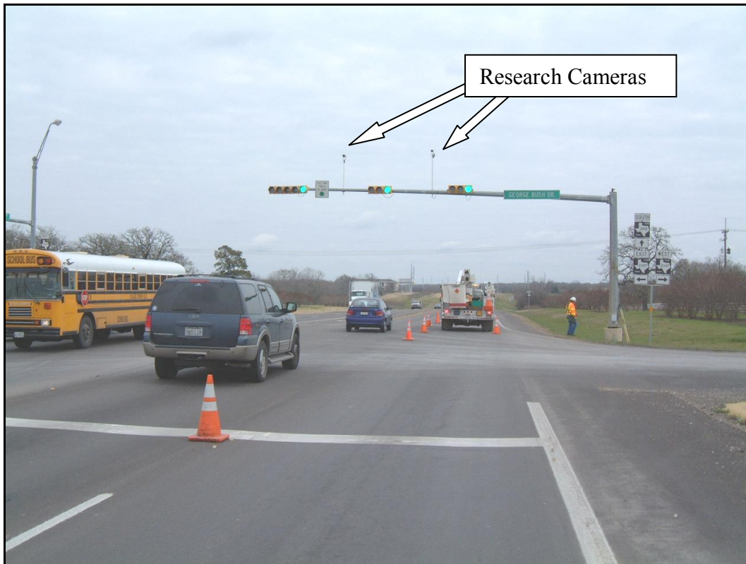
Figure 13. Picture of Signal Heads and VIVDS Cameras for Initial College Station Site.
