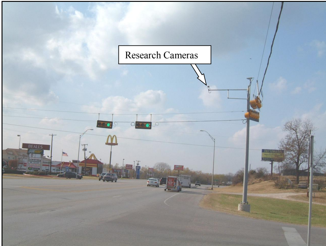
Figure 11. Picture of Signal Heads and VIVDS Camera for Elgin Site.
