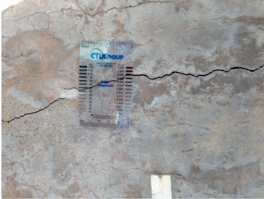
Figure 3-9. Larger Longitudinal Crack Width on Specimen LSC4.
