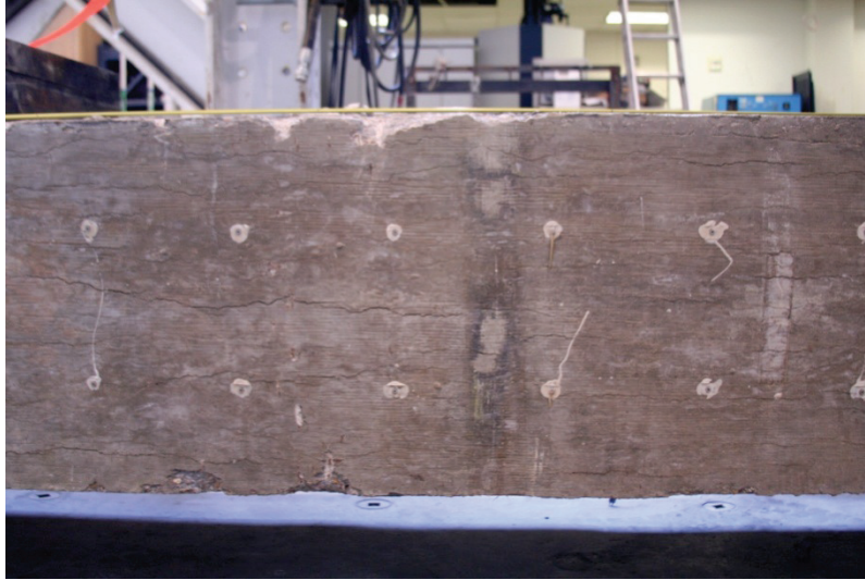
Figure 4-1. Cracking of Specimen #1 prior to Structural Load Testing.
