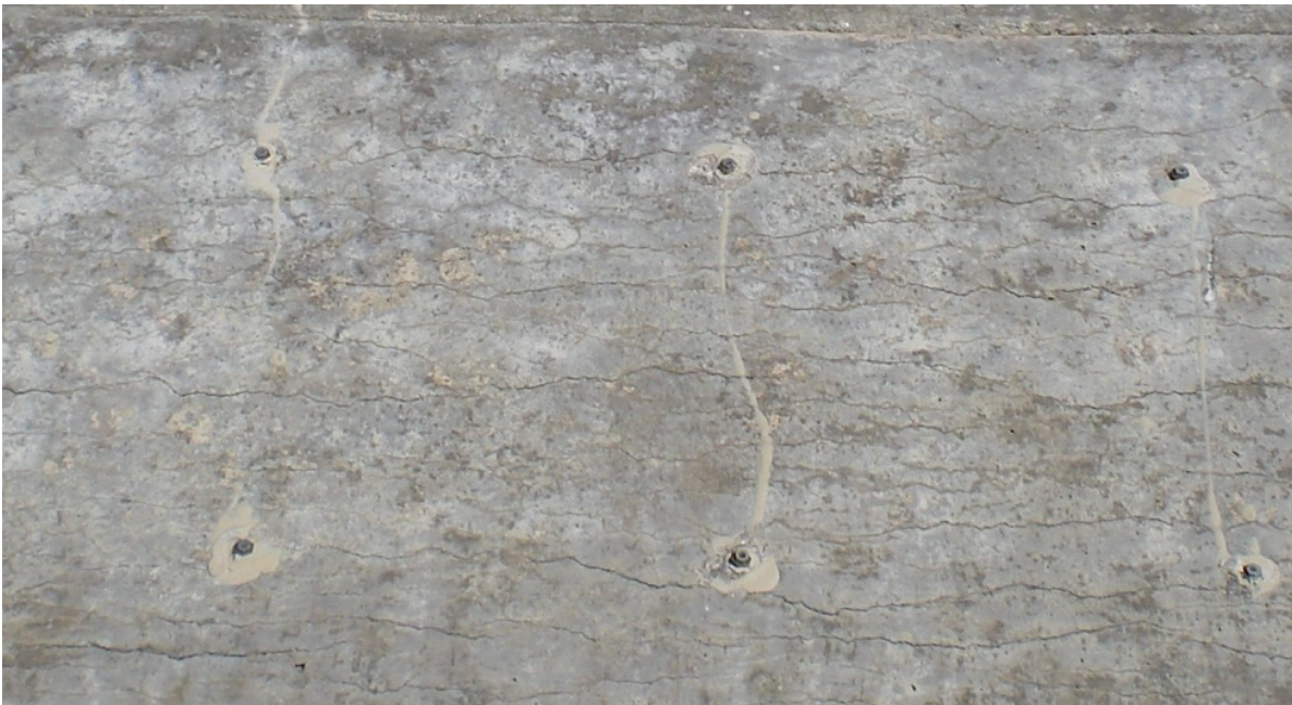
Figure 3-8. Typical Longitudinal Crack in Specimens.
