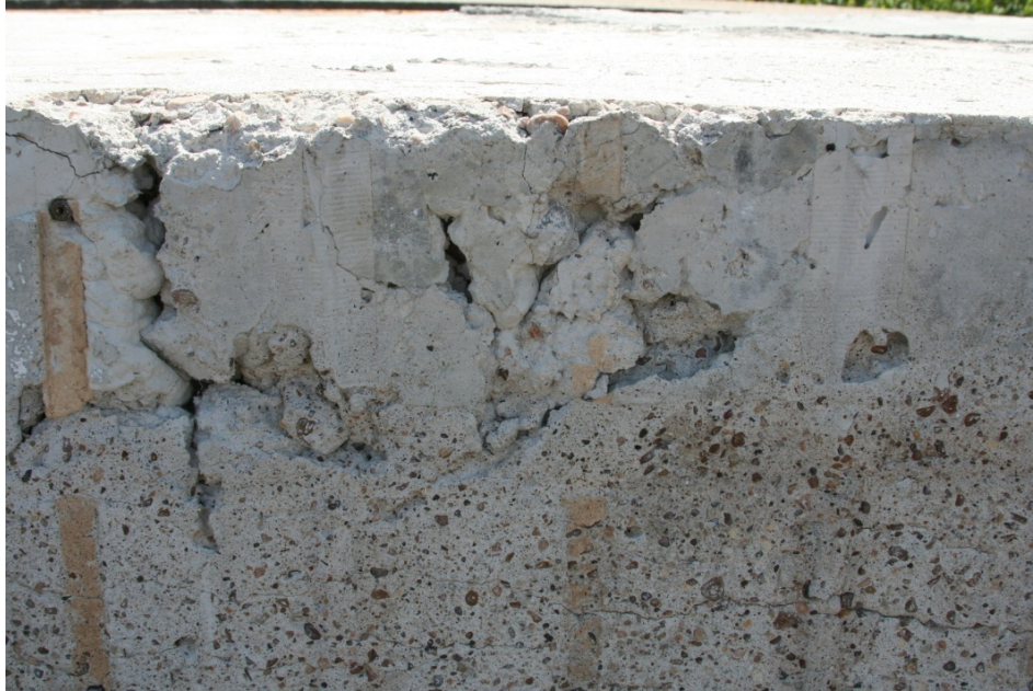
Figure 2-11. Voids in the First Trials.
