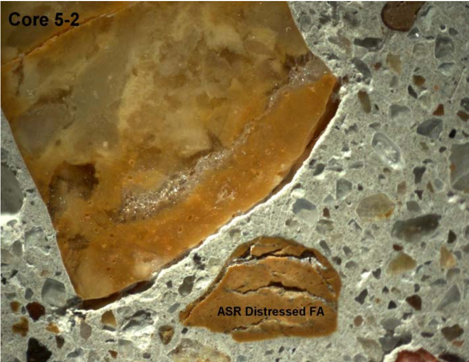
Image illustrating ASR distress in intermediate size aggregate
