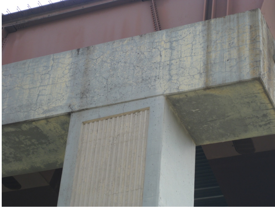
Figure 1-3. Cracking in Bent Cap under Minimal External Loading (Houston, TX).
