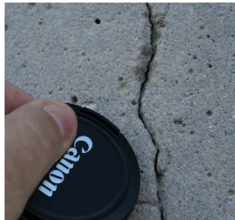
(b) Close-up View of a Typical Crack
