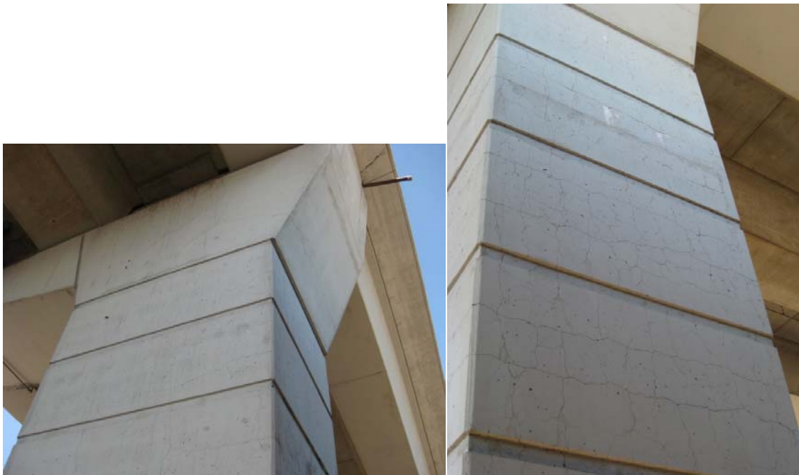
(a) Elevation View and Typical Cracking on Tension Face (Houston, TX)
