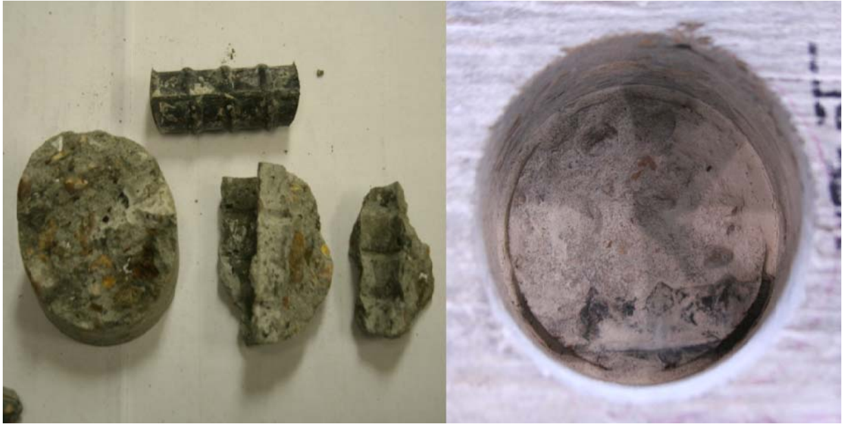
Figure 3-29. Core Extracted above Splice (left) and the Hole from that Core (right).
