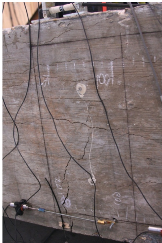
Figure 5-31. Flexural Crack under Actuator 1 during the Four-Point Test for LSC5.
