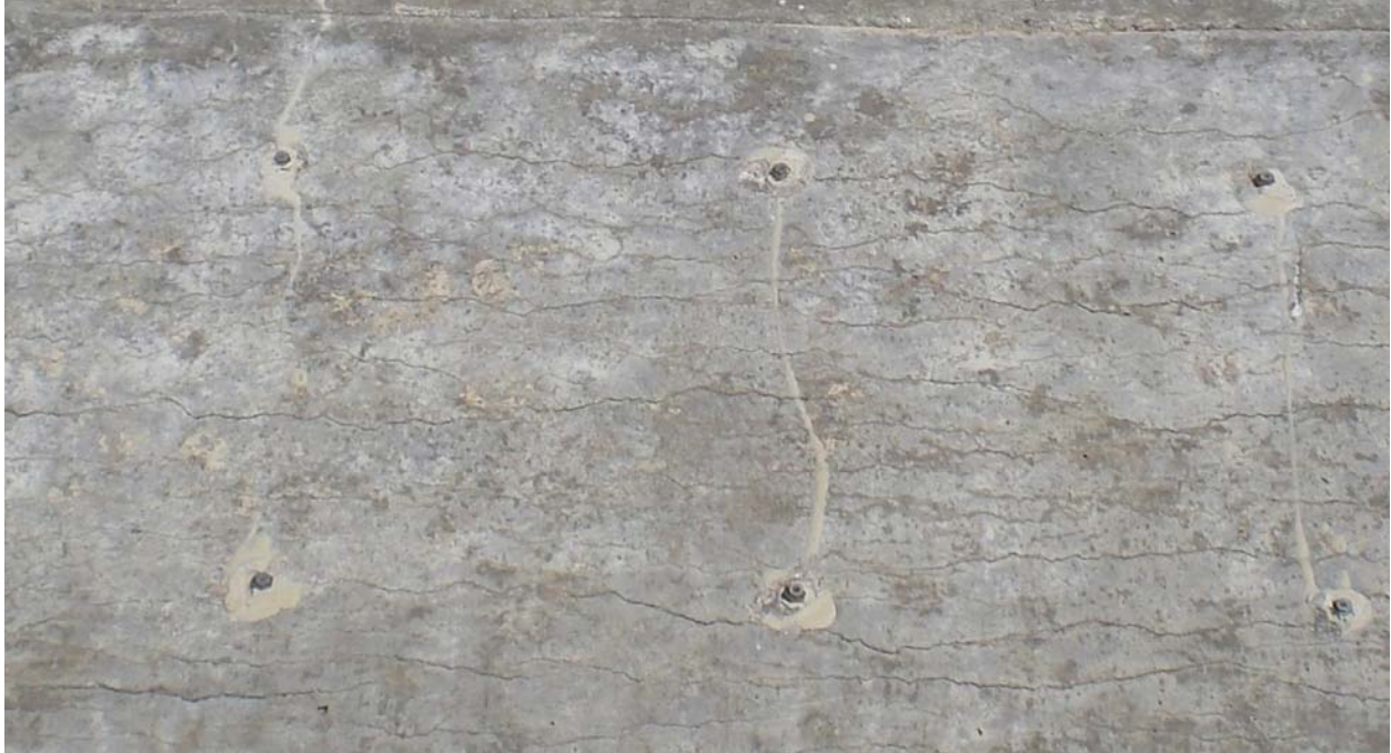
Figure 3-15. Longitudinal Cracks from ASR Expansion.
