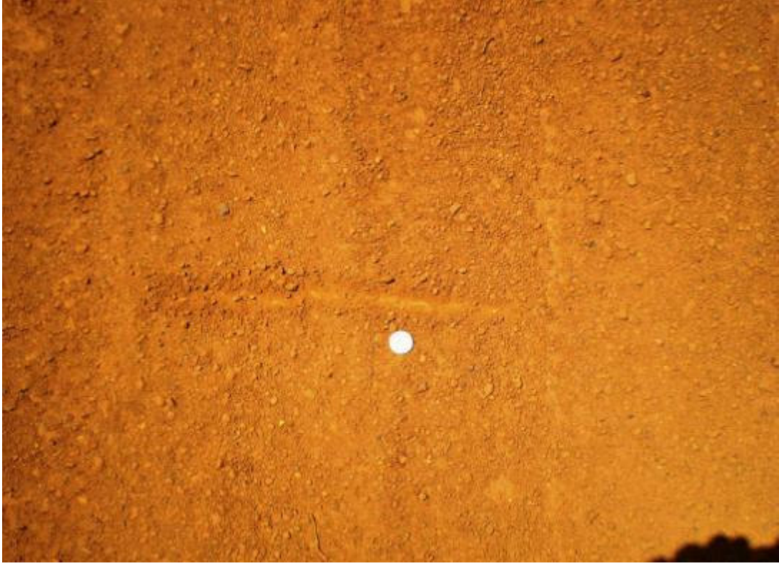
Figure 22. Atlanta, SH 155, MC 30. Loose Material.
