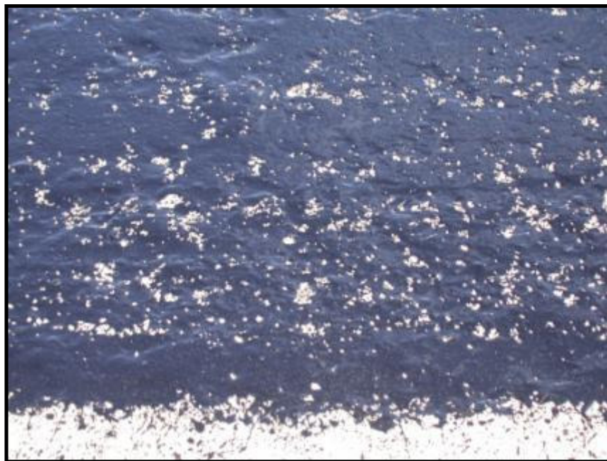
Figure 3. Example of “Freckling” or “Perch Eyes” of Prime Coat on a Dry Base (Senadheera and Vignarajah, 2007).
