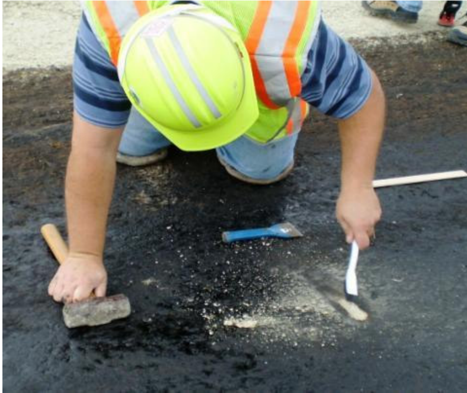
Figure C-4. Penetration Measurement, Showing Chisel, Hammer, and Scale.
