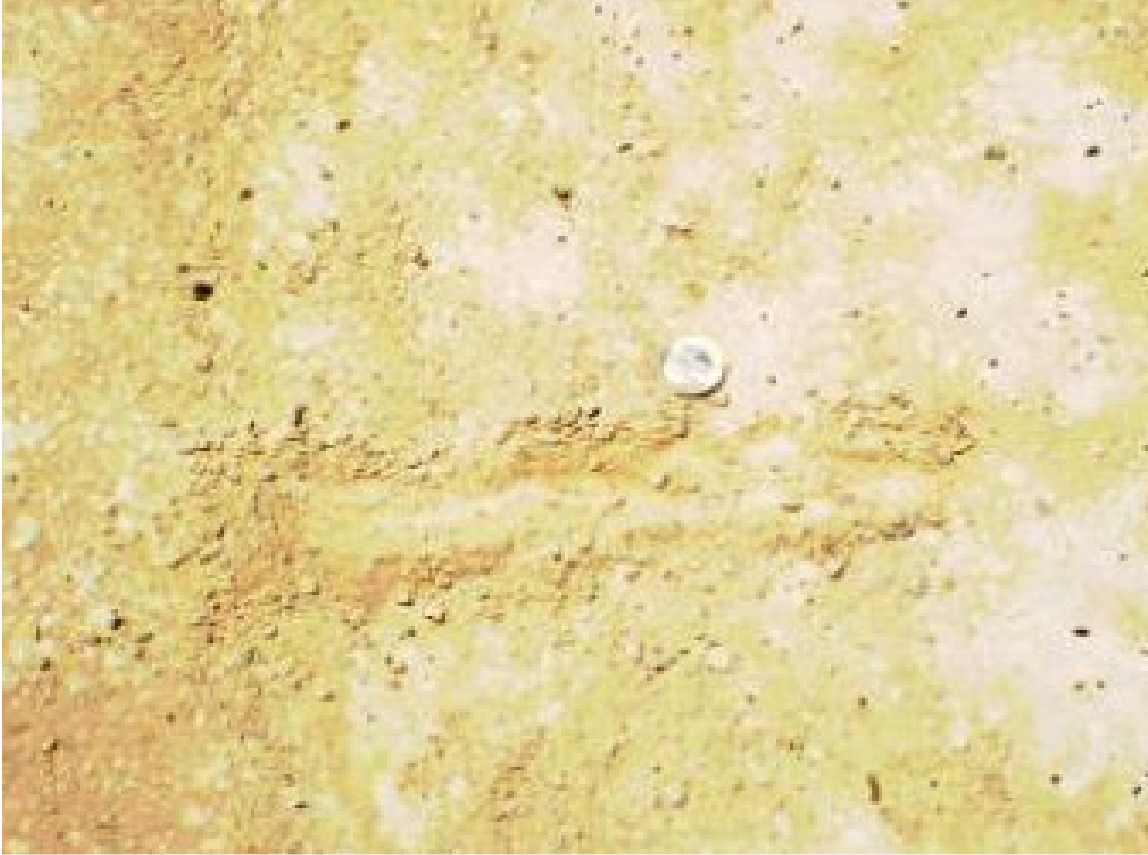
Figure 24. Abilene, FM 1235, AEP. Some Loose Material.
