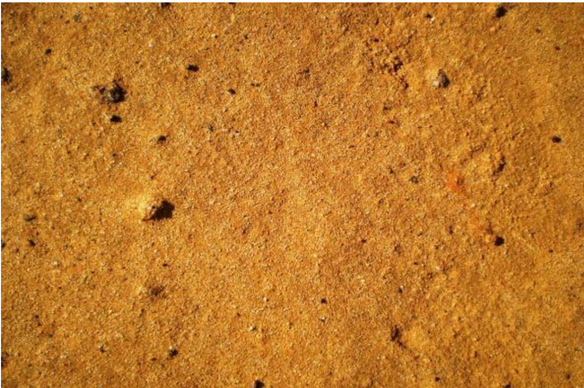
Figure 17. Atlanta, US 59, MC 30. Loose Fine Material.
