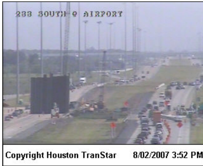
Figure A-11. Right Lane Closure for SH 288 Southbound; Left Lane for SH 288 Northbound.
